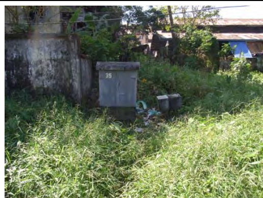
Pic-12: In South-East side of Yangon central station of signal boxes. Garbage and wastewater are seen. Installation environment is very bad.
