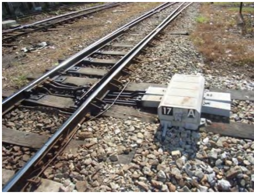
Pic-19: Equipment of interlocking(Germany). It has been used since 1970. At Pazundaung station, there is not the submergence.
