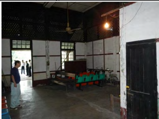
Pic-41: At Pyuntaza station, a spare room is remodeled to signal equipment room and TMS station device is installed.
