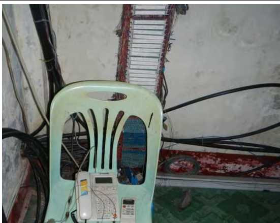
Pic-29: In Yangon central station communication equipment room. Cables are laid from here to the new signal cabin.
