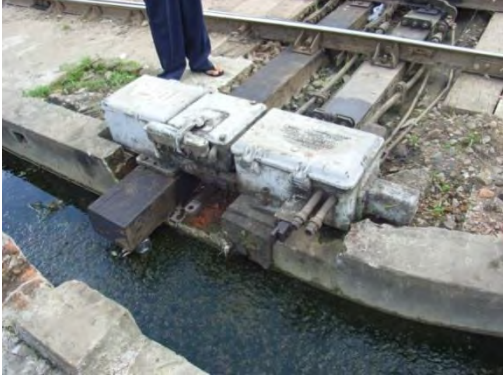
Pic-7: Equipment of interlocking(Great Britain). It has been used since 1950, while repairing it.
