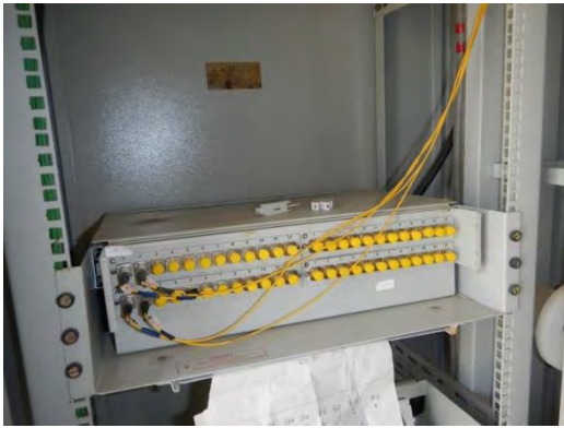
Pic-45: End of terminal rack of optical cable. Optical cables from all TMS devices gather for the rack.
