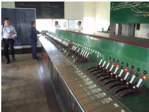
Pic-3: Signal cabin of the Yangon central station. A couse-constituting is operated with levers.
