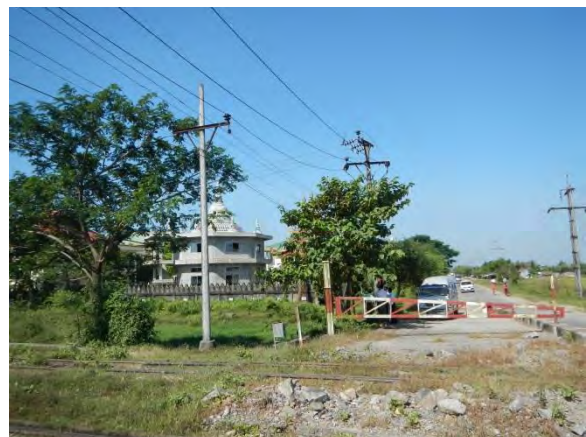
Pic-36: power lines are near the installation schedule of the barrier. There is possibility of contact of power line and the barrier.
