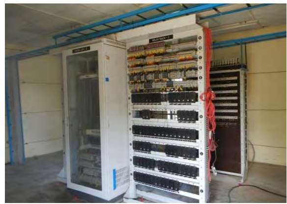
Pic-40: Installation construction of SSI currently performed at the station in which TMS station device is installed (Laydaungkan station)
