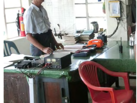
Pic-28: Communication equipment in Yangon central station signal cabin. Cable laying is necessary for the new signal cabin to transfer facilities.
