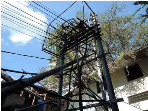
Pic-25: In Yangon central station, the existing supply of electric power track is seen in the depths. A power supply is supplied from YESB power room.
