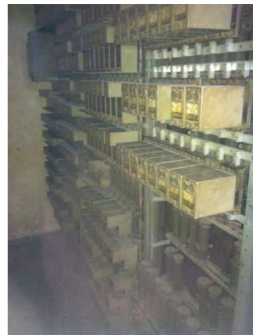
Pic-18: State in the signal equipment room. A difference from Yangon central station is that there is middle track relay.
