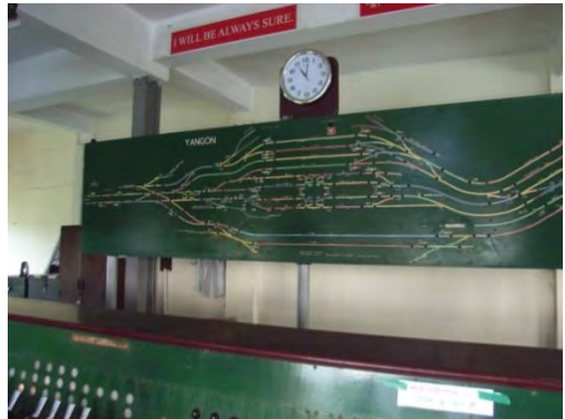
Pic-4: Indicator panel in the signal cabin. The panel informs train on-rail in the station track. Pazundaung station is out of the range.
