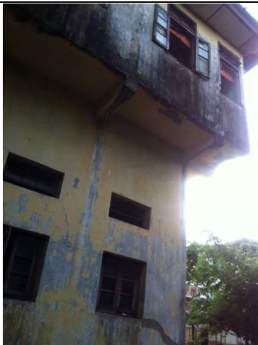
Pic-17: The appearance of Pazundaung station main building. Upper floor is signal cabin, and lower floor is signal equipment room.
