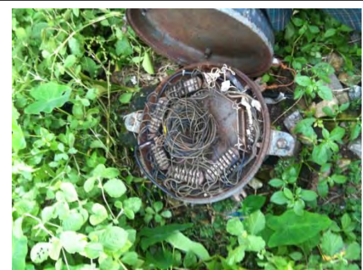
Pic-22: Unlike Yangon central station, there is only the connection box in near the track. This is a horizontal connection box
