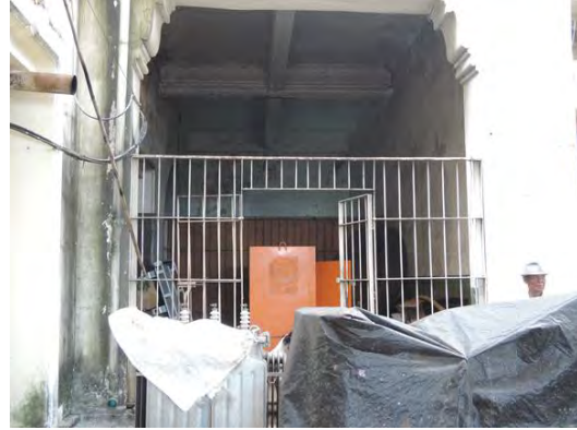
Pic-26 An existing spare power supply is on the east side first floor of Yangon central station main building.
