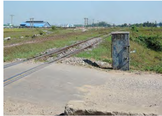
Pic-38: There is a subterranean electric wire of 600v near Kyang Sit Thar level crossing. And the power receiving box has a terminal.
