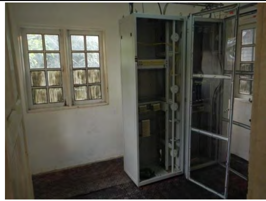
Pic-44: TMS central device and station device are connected with the optical cable. The network is built through the rack.
