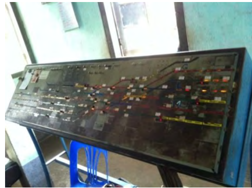
Pic-16: Indicator panel in the signal cabin of Pazundaung Station. It has been used since 1970. The station has 18 routes.
