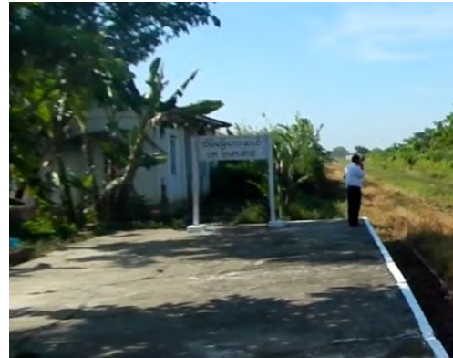
Pic-46: Since there is no rack in Eimshaylayse station, connection with existing optical cable is required.
