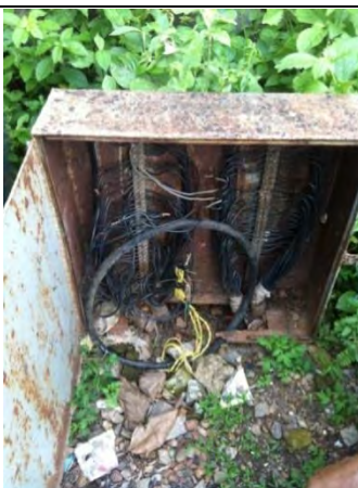
Pic-23: Vertical connection box. Cable is buried directly and only end leaves from the ground.
