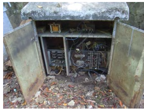
Pic-10: Wayside signal box. In the box, there are relays for train detection. The state is not good by influence of flood.
