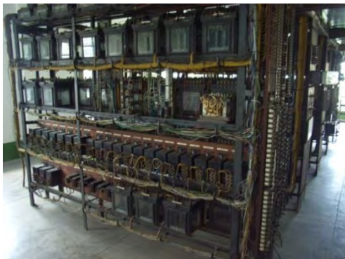
Pic-5: Signal equipment room. Relays and cables are used since 1950.
