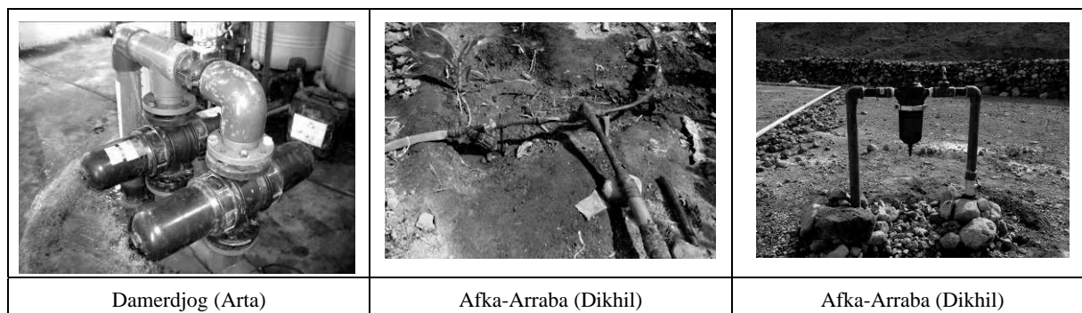
Figure 7.4.3 Case examples of the screen filter installed in Djibouti
