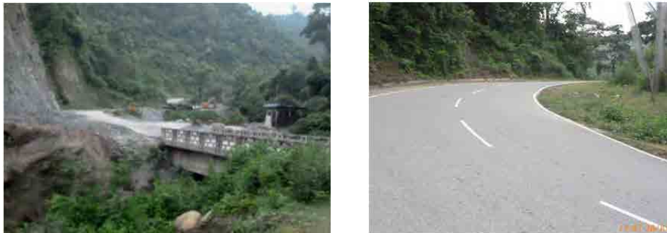
Source: Photos taken by JICA Study Team (Left) Section being widened, (Right) Widened section <Figure4-3> Condition of PNH3
