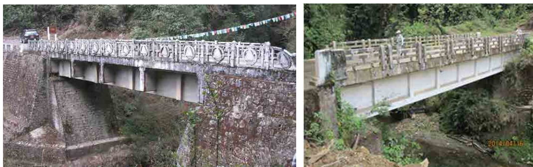
Source: JICA Study Team <Figure5-3> Deteriorated bridge on PNH-1 (Nagni zam Bridge) and PNH-4 (Chaplekhola zam Bridge)
