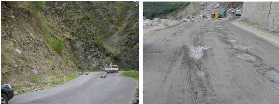
Source: JICA Study Team <Figure 4-5> Present condition of PNH-5
