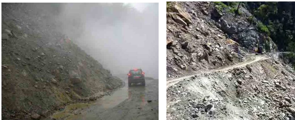
Source: Photos taken by JICA Study Team <Figure4-4> Slope failure condition (PNH4)
