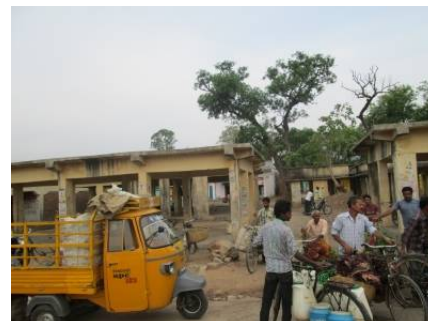
Unused sheds in Pithauria Market Source: JICA Survey Team
