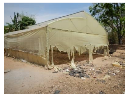
Poly nursery house torn by swine Source: JICA Survey Team
