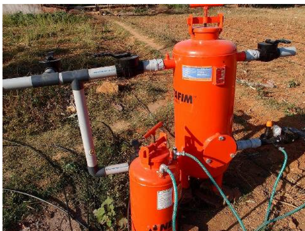
MDI Facility of Direct Pumping Type (Hazaribagh District)
