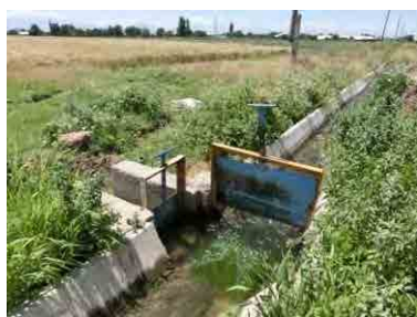
Tertiary canal (concrete flume)
