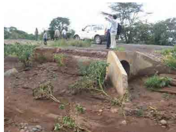
Access road destroyed by floods in Ruiru Area
