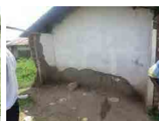
A house seriously damaged by floods
