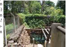
Example of slope protection using Gabions. Situated at the Intake works for Taveta Water Supply adjacent to Njoro Kubwa Springs
