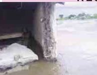
Flood damaged house in Nyora
