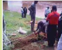
WRUA members dig trench to lay in cabling pipes that links the gadget at the river and alarm at observer's house
