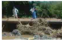
Debris and obstacles along the river channel
