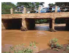
Bridge marking the boundary between lower and upper Lumi. The upstream side of the bridge is usually dry during the dry season. In wet season high flows from Mt. Kilimanjaro causes flash flooding
