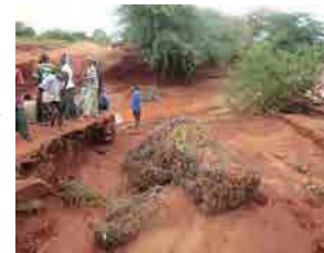
Bridge on Gully in Rekeke Village swept away by flood waters
