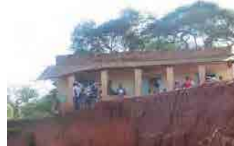
Masaini gully that continuously enlarges due to heavy soil erosion as a result of the flash floods and currently has damaged part of a permanent house structure that is near
