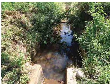
Silt Trap to prevent excessive deposition in reservoir
