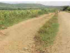
Murrum road which flood water flow on
