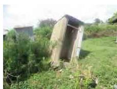
Almost collapsing toilet facility
