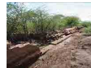
Concrete Wall dyke broken after being hit by flash floods in Laitoktok-Taveta Road
