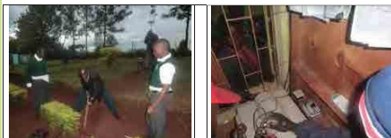
Description : Teachers and students participate in the installation of the rain gauge and the sensor Description : The sensor having been installed is being tested and also explanation to the observer on how to operate and manage the sensor
