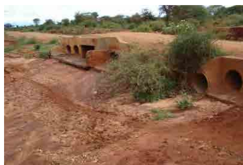
Bridge with pipe culvert installed at the dry up river crossing the road
