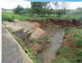
River Bank erosion before bank Protection
