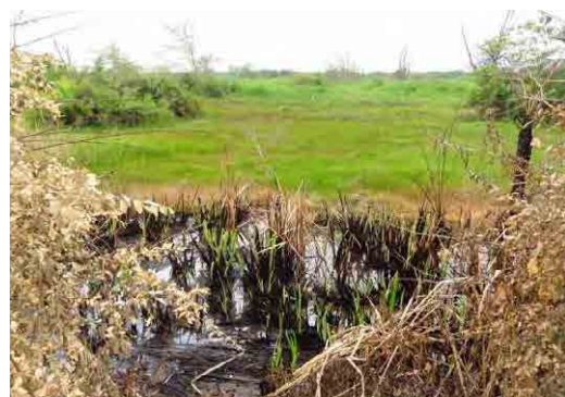
Damp ground where the bank of Canal-C has been washed out
