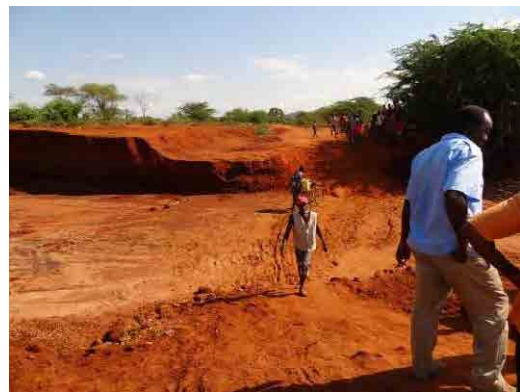
Road Bridge rushed out Place : Rengesa
