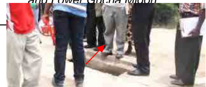
Vandalized culvert slab pavement
