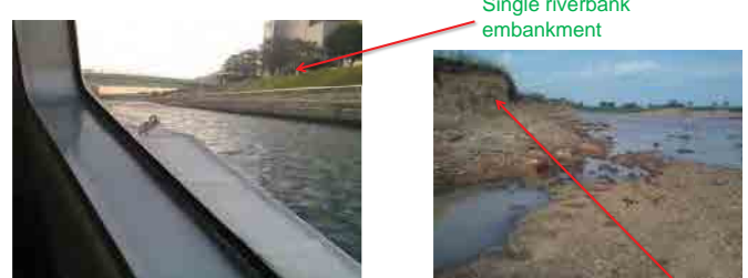
Current status of damaged riverbank at R. Gucha Migori
