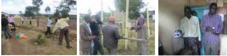
Installation process of rain gauge for CBFews
