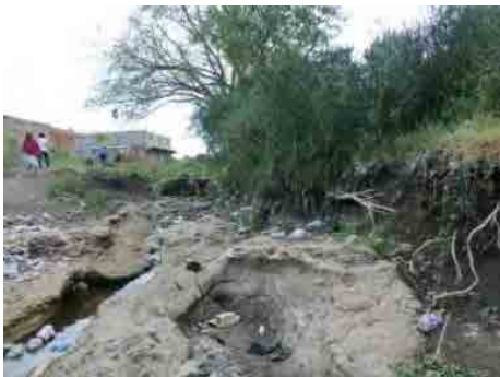
Bank erosion near urban area
