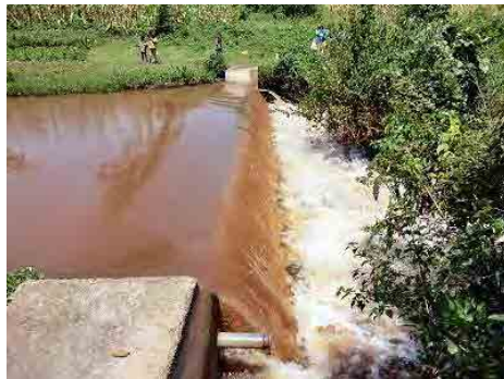
Check Dam (Example of Nzoia River)
