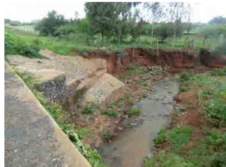
Bank erosion at the Eastern Marania River
