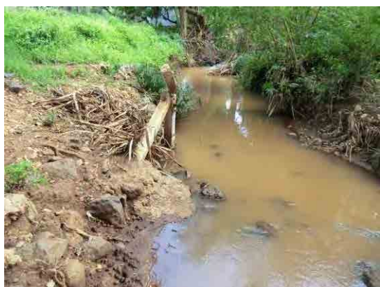
Water Level Gauging Station No. : 5DA04 Observation River : Eastern Marania River Special Note : Water level gauge is broken off and damaged.
