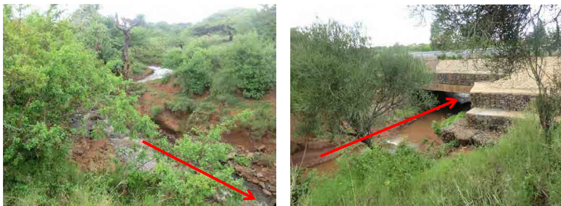
Photo 4.1.1 View of Upstream from the Crossing Point of Highway A2 (Left: View of upstream from the bridge, Right: View of bridge from upstream)
