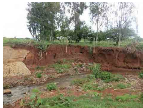
Progressed river bank erosion in Eastern Marania River Place: Upstream of Isiolo River
