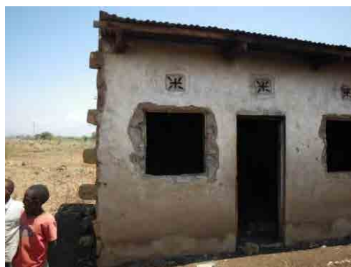
House was destroyed by flood
