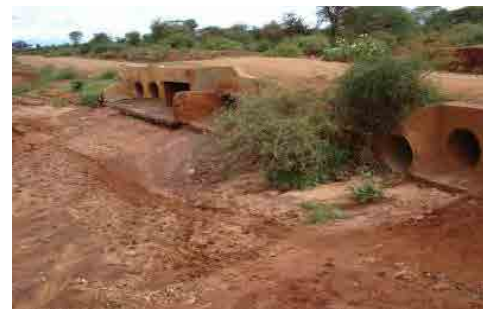
Bridge with pipe culvert installed at the dry up river crossing the road
