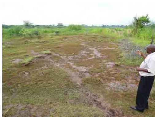
Photo 3.1.2 Broken point of the embankment Canal-C
