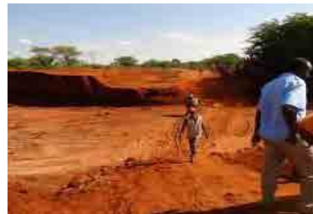
Washout of the concrete bridge of the same structure to the above by flash flood Place : Rengesa
