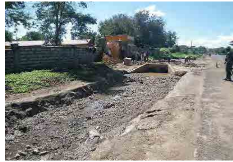
Very few drain channel installed in the urban area (Place: Isiolo Town)
