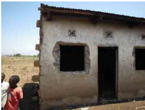
House was destroyed by flood
