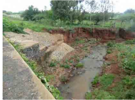
Bank erosion at the Eastern Marania River
