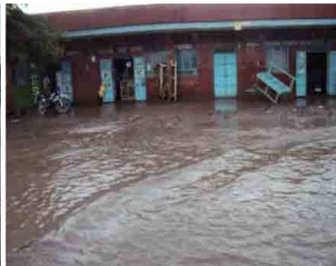
Situation of inundated house
