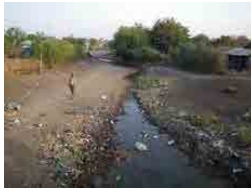
Downstream of Merire River (upstream view) squatter's houses are on the left bank of the river channel
