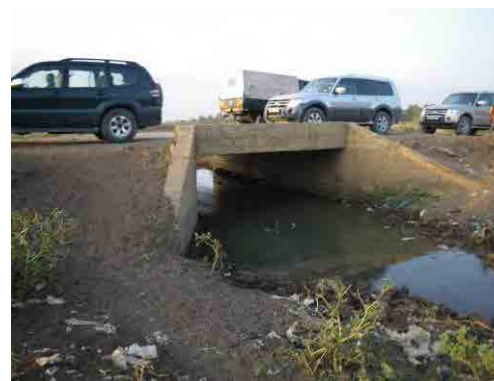
A box culvert bridge at the downstream end of the town of the Merire River (Downstream view)
