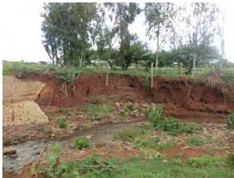
River bank erosion along Eastern Marania River (Place: Upstream of Isiolo River)
