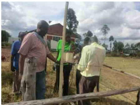
Installation of a rain gauge and sensor at Emuria Dikiri Secondary School
