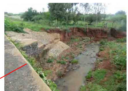
Eroded bank before protection
