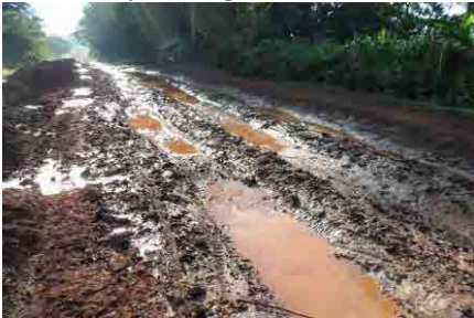
Identify damaged road section
