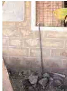
Wire between gauge and battery
