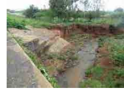
Bank erosion at the Eastern Marania River 44
