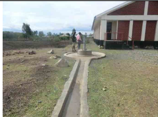
Description : CFMO at Kanyango has managed to install a 60M deep borehole with a handpump at EVC
