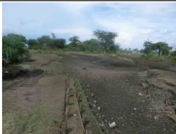
Description : Weir is silted and community members have not remove the silt inspite of the dry season leading to overflow of water
