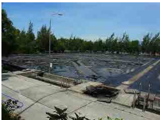
Ngu Hanh Son WWTP (Anaerobic Lagoon)
