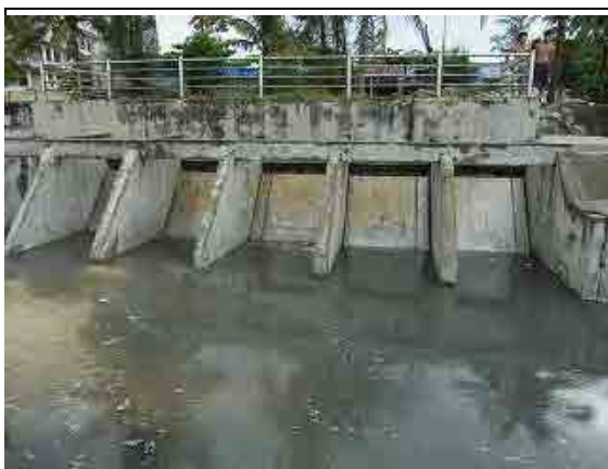
Overflow Water from Pumping Station
