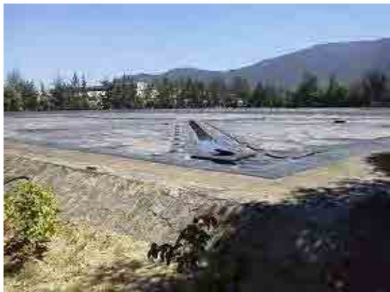
Son Tra WWTP (Anaerobic Lagoon)
