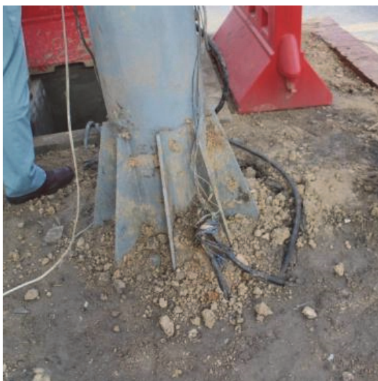
Existing Signal Cable Wiring
