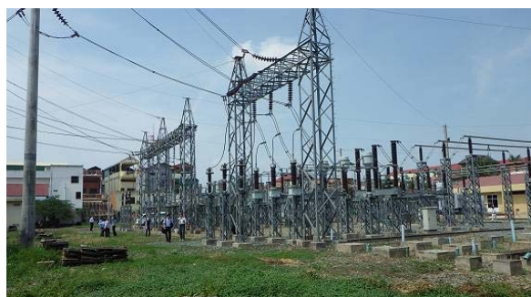
1) 115kV Switchgear installation position
