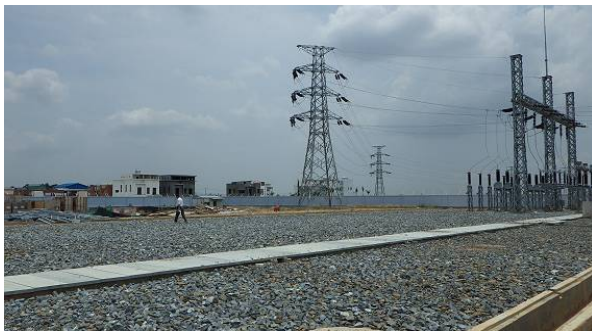
1) GS5 115kV bus north side
