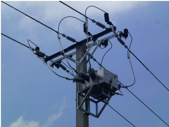
Fig. 8.4-8 Pole Mounted Type Switch
