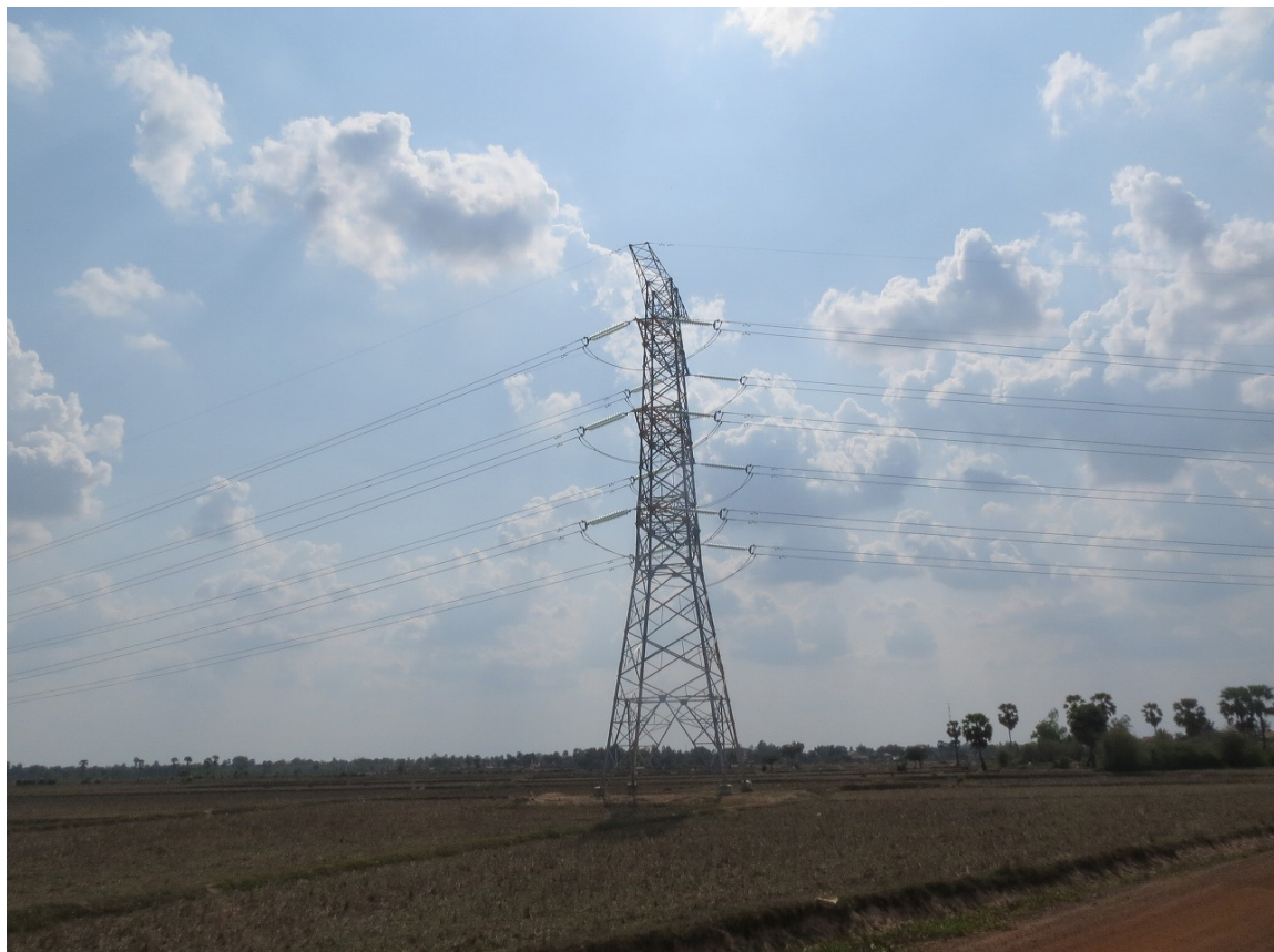
図 8.1-3 230kV Steel Tower in the Midpoint of NPP and WPP
