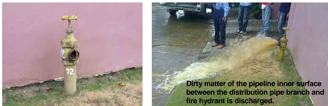
Pict-3.2.3 Surface type fire hydrant (Right: water distributed from a fire hydrant.)
