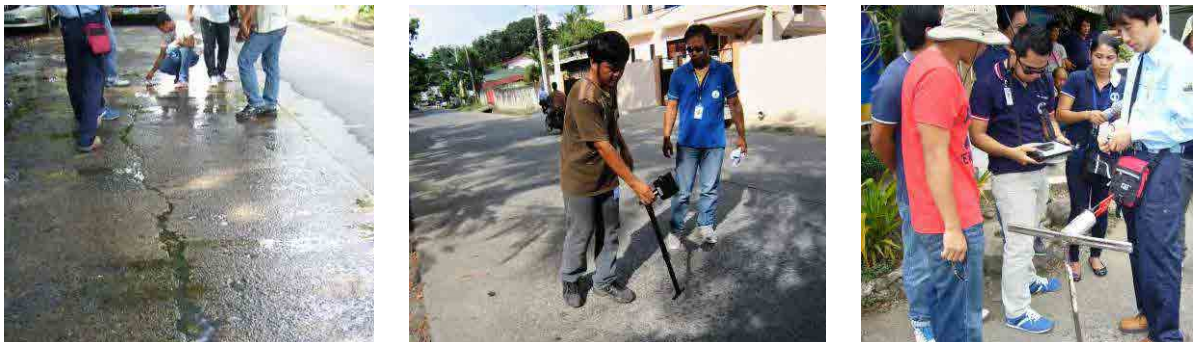
Pict-3.1.1 Surface water leakage occurrence location (Left) / Survey of underground water leakage (Center, Right) [3-2]
