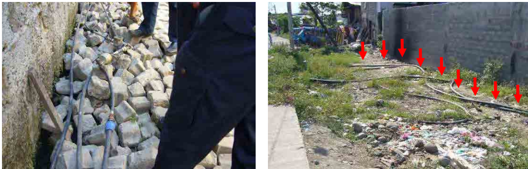
Pict-3.2.5 Illegal connection point (Left) / Exposed PVC pipes that are laid above ground (Right) [3-11]
