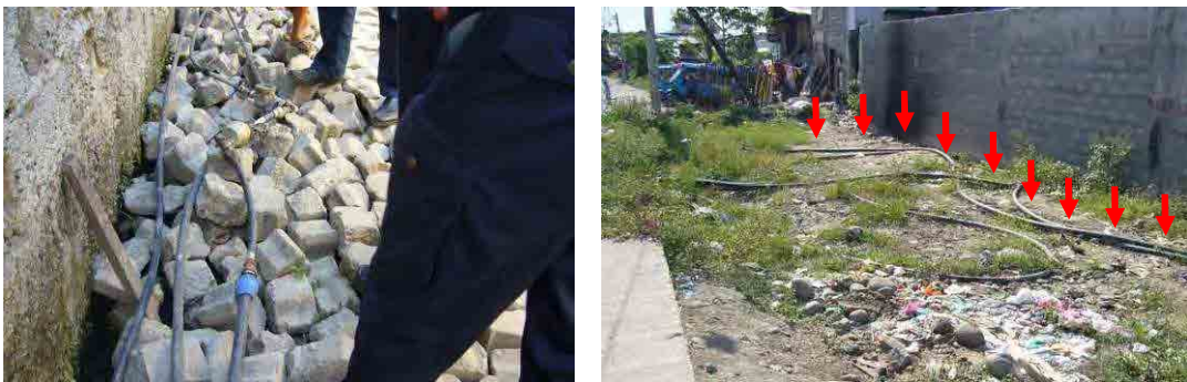
Pict-3.2.5 Illegal connection point (Left) / Exposed PVC pipes that are laid above ground (Right)
