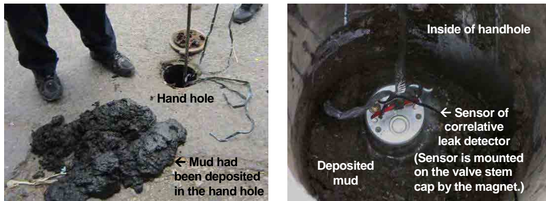
Pict-3.2.2 The inside of the hand hole that has not been maintained
