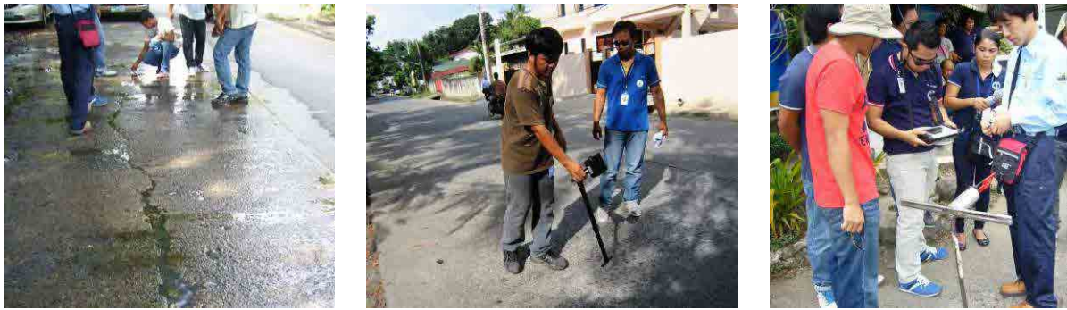
Pict-3.1.1 Surface water leakage occurrence location (Left) / Survey of underground water leakage (Center, Right)
