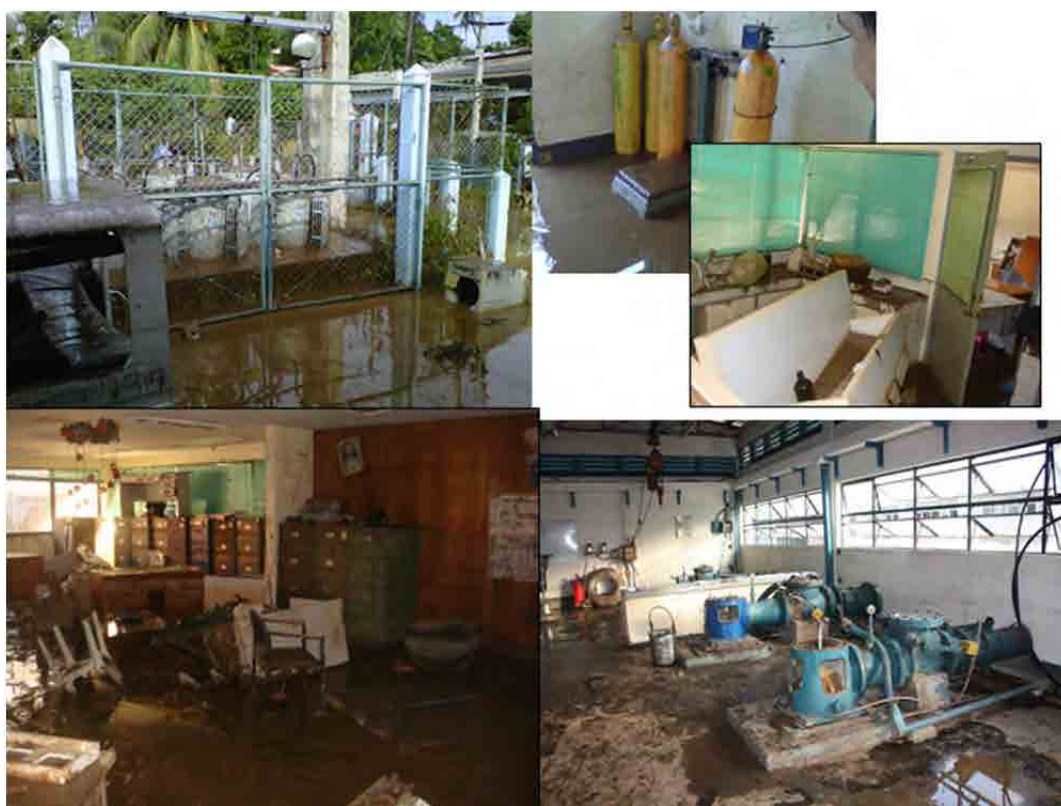
Slide 7-5 COWD’s facilities damaged by Typhoon Washi
