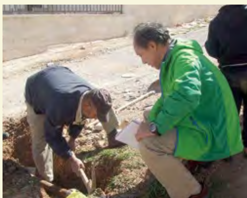
JICA expert checking the condition of a water distribution pipe in the situation analysis on water and sewerage services in host communities.
