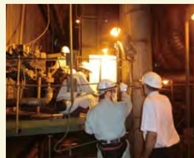
Installing the heat-resistant camera inside the boiler (Photo Credit: Security Japan Co. Ltd.)
