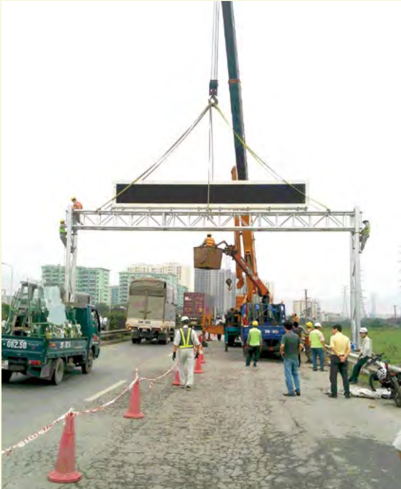
Installing a traffic control system provided under Grant Aid on a highway in Hanoi, Viet Nam.
