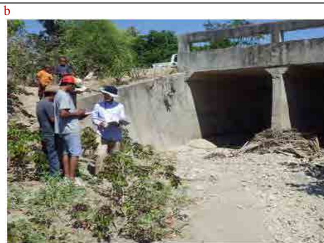
Site Training to C/P how to survey for Updated Bridger Register Database(Seo.2014)
