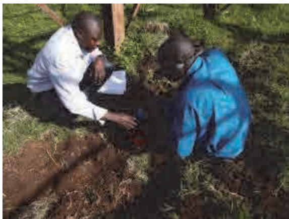
Check of gate valve
