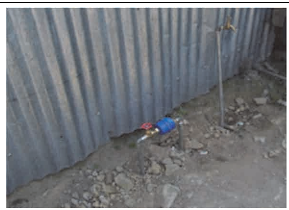
Customer meter after changing to expose from ground surface
