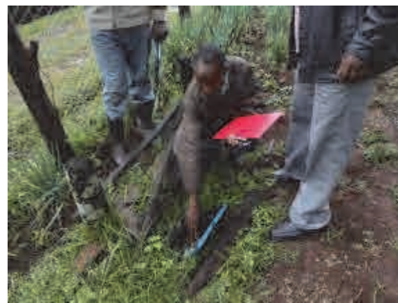
Check of customer meter
