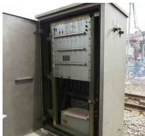
(b) Level crossing control equipment
