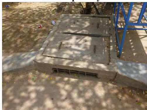
Figure 4.6-11 Inlet of Drainage at KP 393
