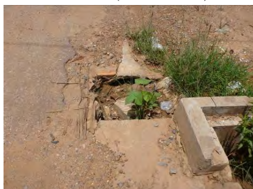
Figure 4.6-4 Clogged Drainage Pipe near KP 186 + 500
