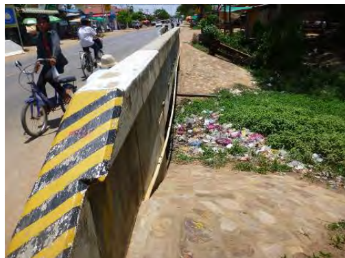
Figure 4.6-2 Telephone Cable on Br. 56 (KP 201 + 800)
