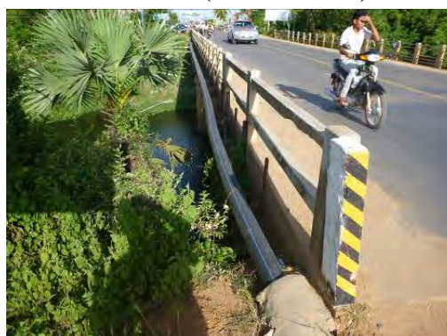
Figure 4.6-3 Water Supply Pipes on Br. 48 (KP 187 + 500)
