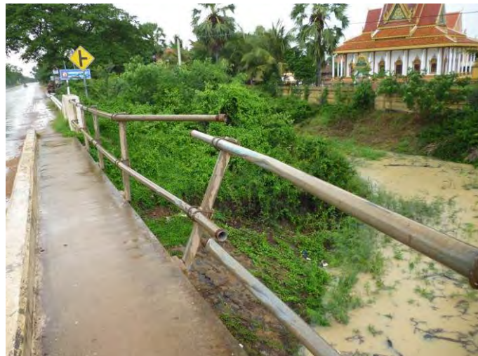
Figure 4.4-4 The Damaged Handrail on Br. 59
