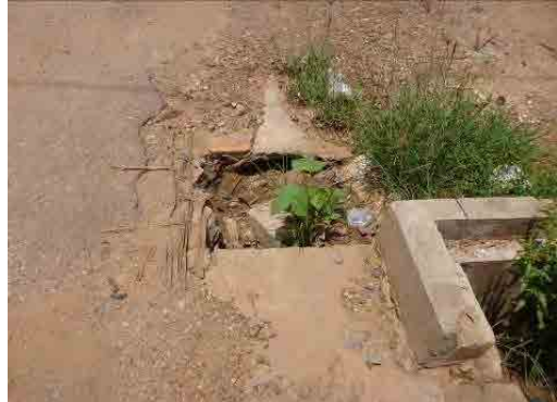
Figure 4.6-4 Clogged Drainage Pipe near KP 186 + 500
