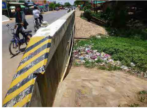
Figure 4.6-2 Telephone Cable on Br. 56 (KP 201 + 800)
