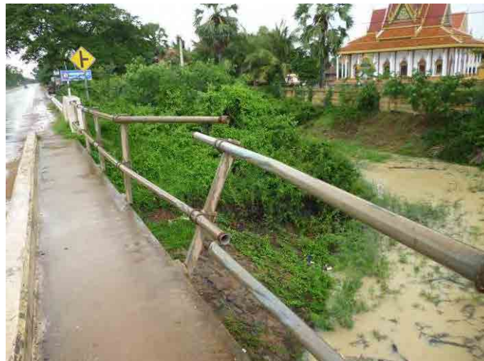
Figure 4.4-4 Damaged Handrail of Br. 59
