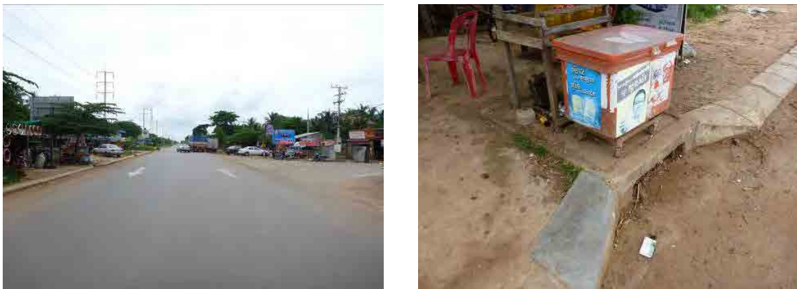
Figure 4.2-6 Road Surface Lower than Adjacent Land in the Commercial Area (Left) and Inlet of Drainage Installed under CRIP
