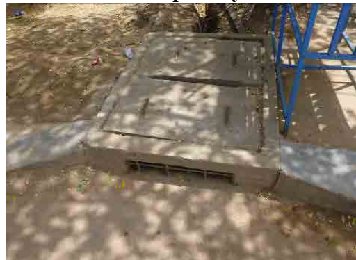
Figure 4.6-11 Inlet of Drainage at KP 393
