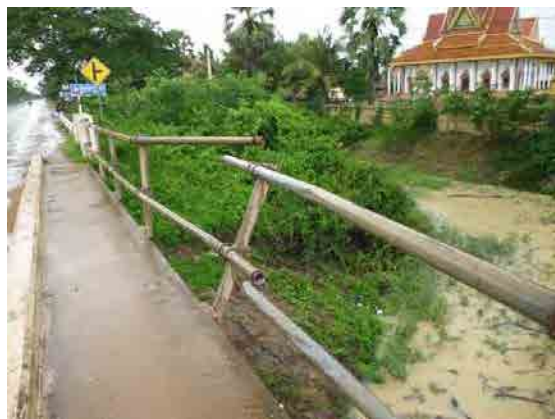
Figure 4-7 Damaged Handrail of Br. 59
