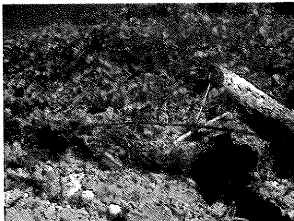
Photo 5-8 Broken shore protection with broken wires
