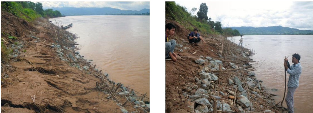
Photo 3.5-2 Deformation of Slope Protection Work and Monitoring Activity by C/P Officials
