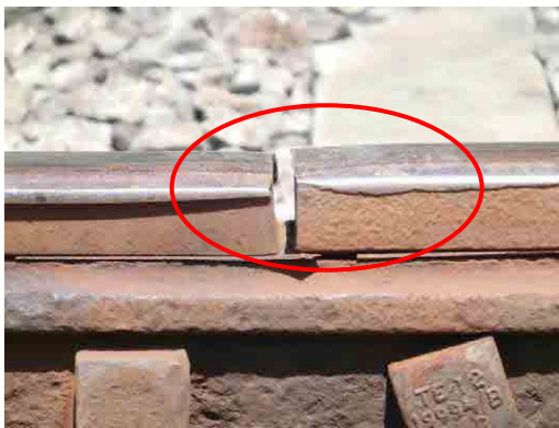
Figure 1.6.3 Deformation of Rail
