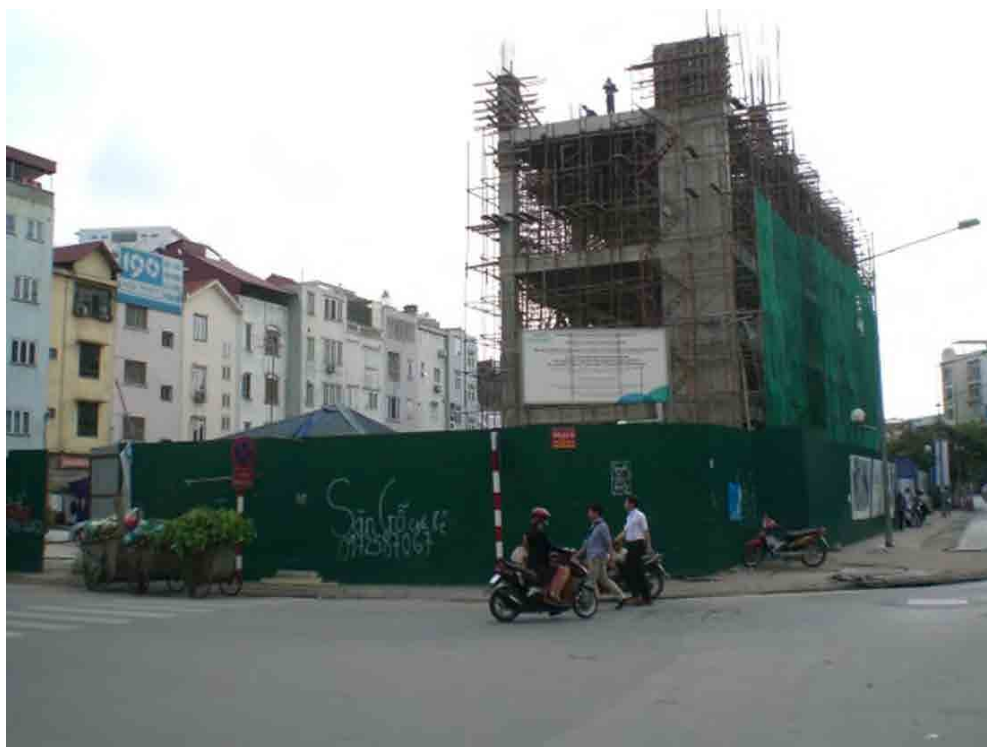
Figure 3.5 Construction site of Kim Ma BRT Terminal Source: Study team (taken on Jun 30, 2014)
