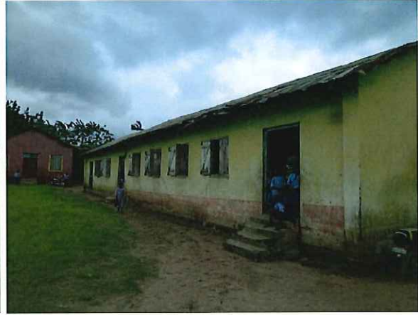
P10-N25 ST. PHILIPS PS, FASOLA (Deteriorated building)
