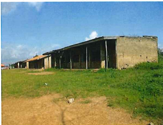
N4-P4 IMG PS Olubadan (Deteriorated building)
