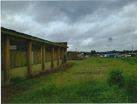
P22-N39 BAPTIST PS, MAYA LANLATE (Deteriorated building)
