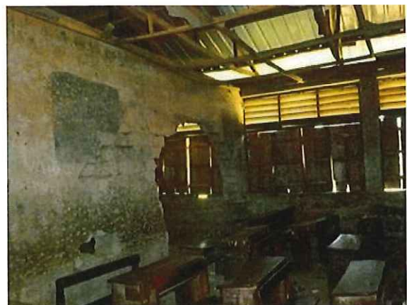
N4-P4 IMG PS Olubadan (Deteriorated classroom)
