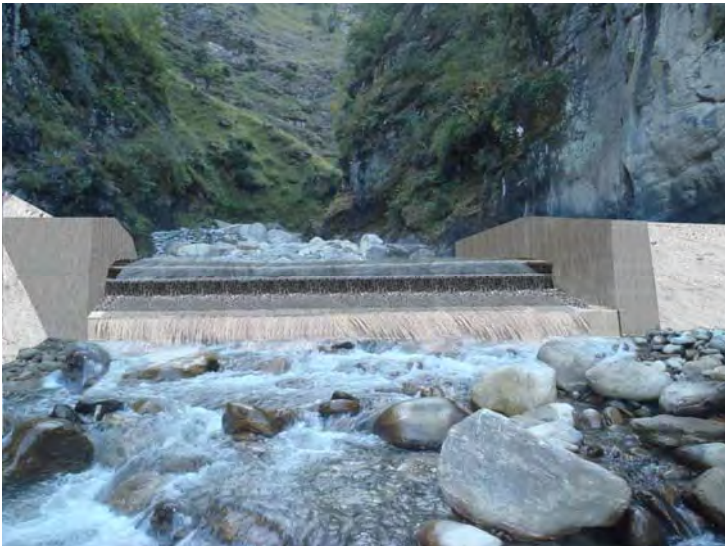
Bajura Micro-hydropower Plant Intake
