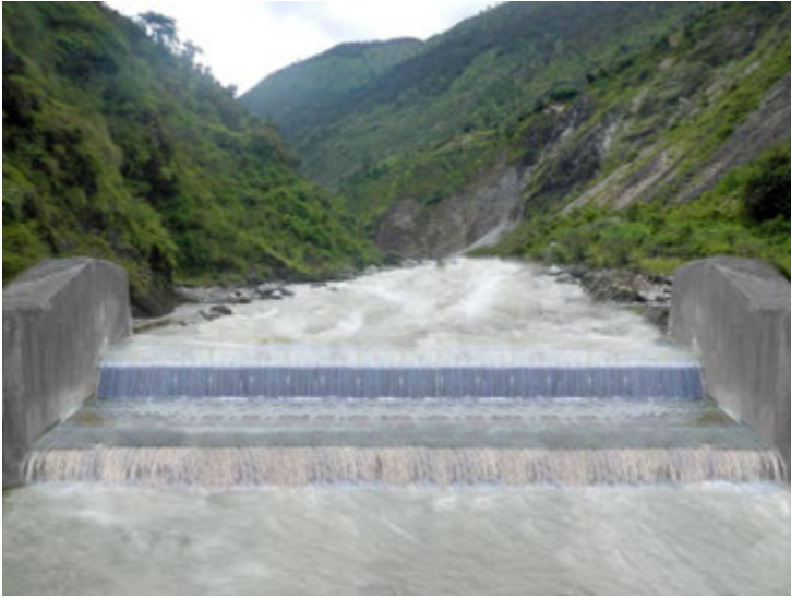
Bajhang Micro-hydropower Plant Intake
