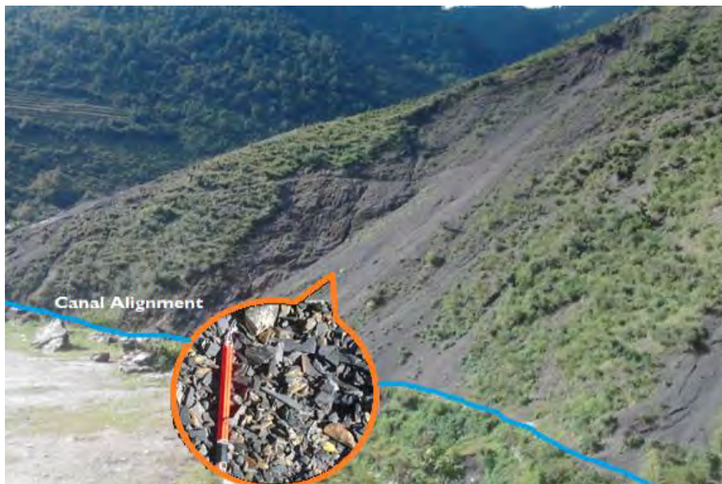
Figure 7-9 Highly Disintegrated Rock between Chainage 0+185 and 0+420
