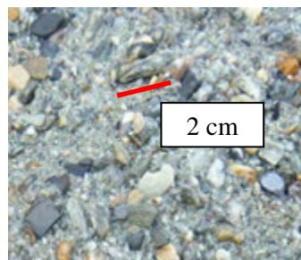
Figure 1-7 Sand deposited in the existing headrace channel (near intake)
