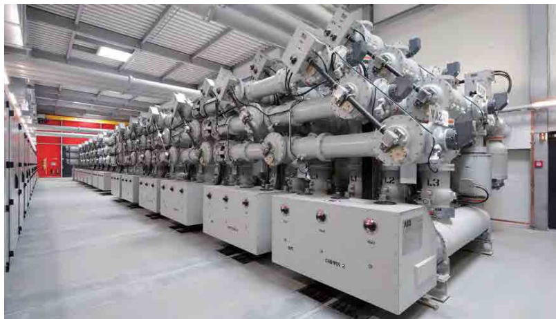
Figure 3-4-31 Example of GAS insulated switch used in indoors
