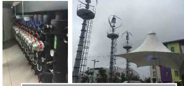
Geothermal system piping & wind turbines
