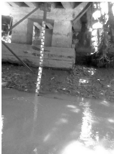
Water Level Post of Kyaek Hta Water Level Gauge Station
