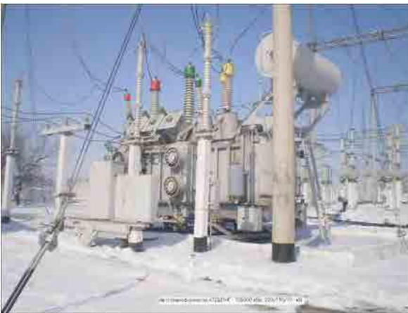
(c) The existing transformer
