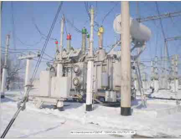
(c) The existing transformer
