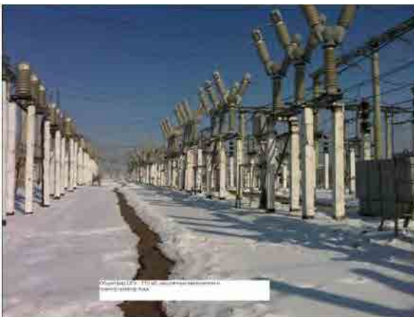
(e) The existing 110kV Switchgear Yard
