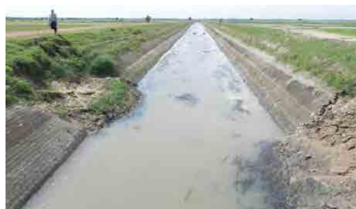
Collapsed canal bank by cattle moving
