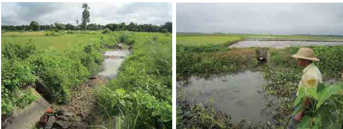
Left: an outlet installed at a North Nawin distributary canal, which does not have gate but 15” pipe only, after which there is tertiary canal managed by farmers. Right: an 18” outlet installed at a Wegyi distributary canal providing water directory to the neighbor paddy field.
