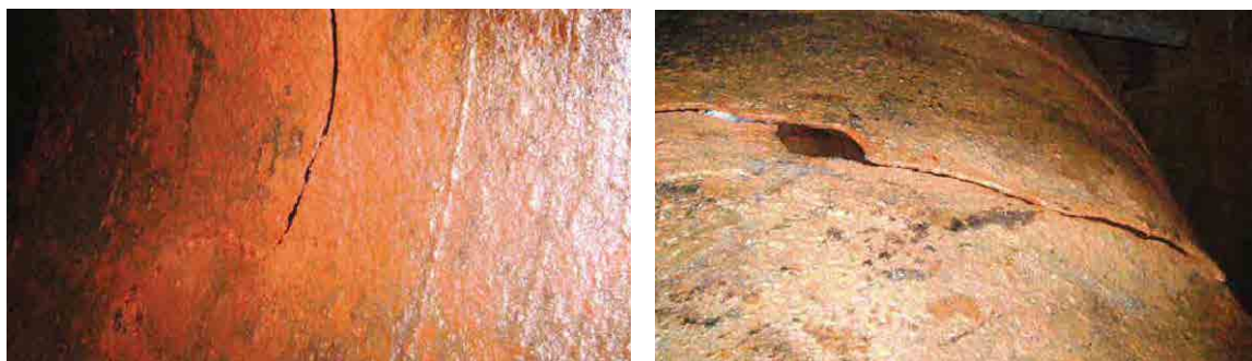
Steel Pipe Crack of Inside-view (left) and Outside-view (right) along Outlet Pipe of the Intake
