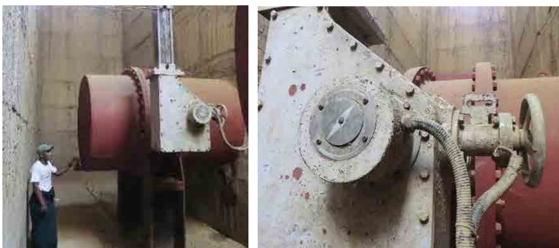
Present Situation of Inlet Valve placed for Suspended South Nawin Hydroelectric Power Plant
