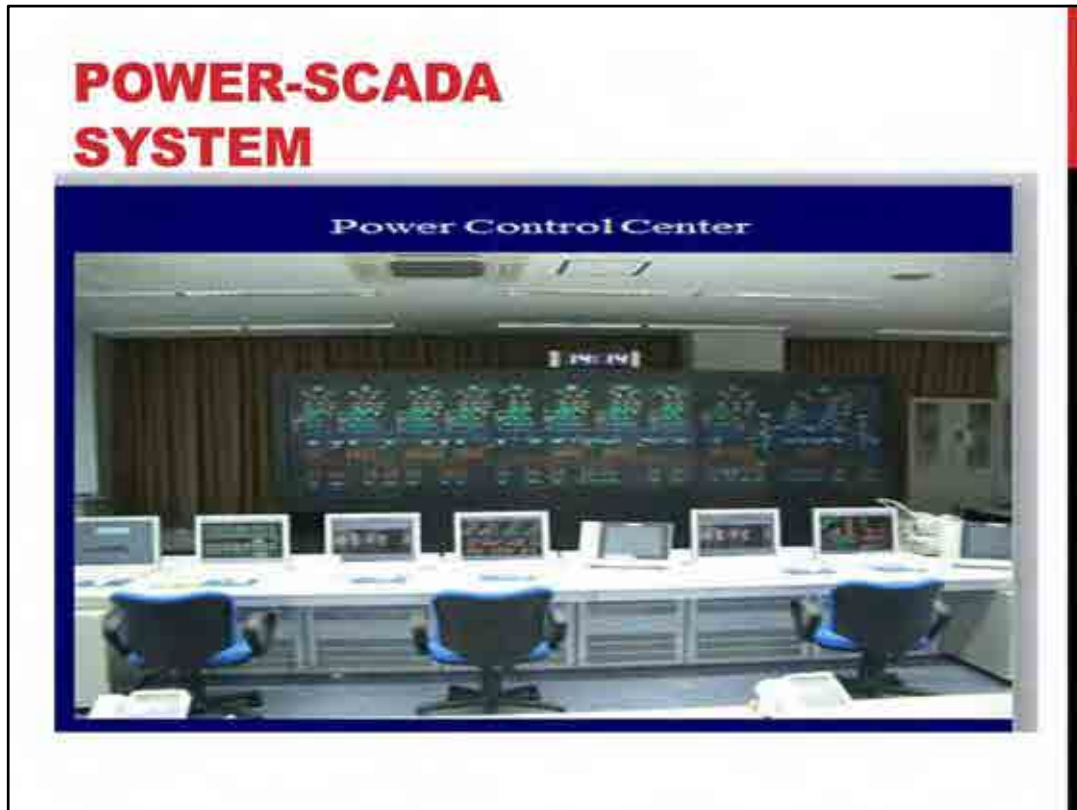
This is the picture of dispatcher desk for Power-SCADA system for a Japanese Shinkansen.
