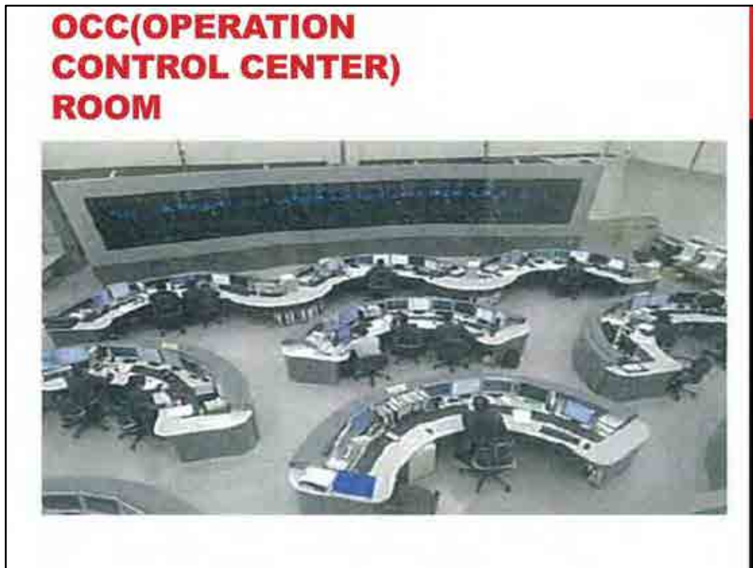
This is the image of Operating Control Center room.
