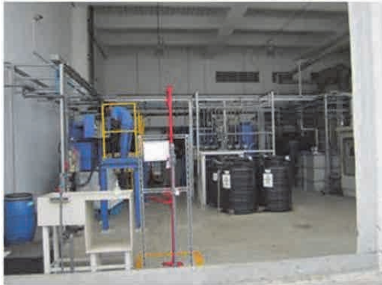
Effluent treatment equipment
