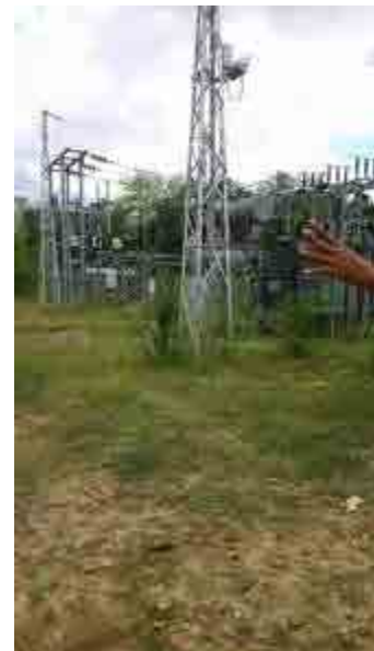
Substation (1) in Nyaung-U Town
