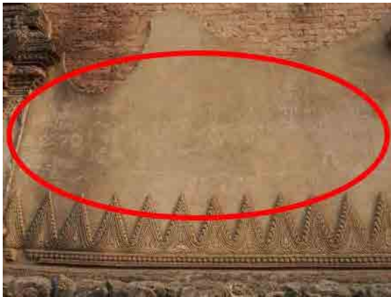
Graffiti on stucco wall
