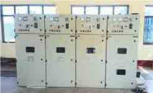
Substation (2) in Nyaung-U Town There are new feeders.
