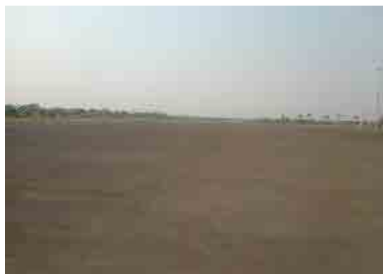
Pavement of airstrips has been deteriorated. Visual flights are assumed.
