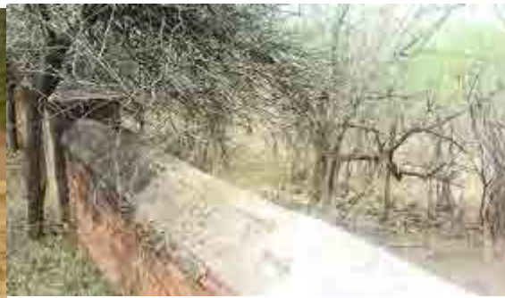
Holding basin on the other side of the brick wall that uses gradient of land topography. The mechanism is very natural: water flows into the reservoir after being filtered by porous rocks.
