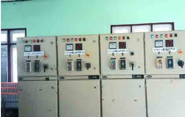
Feeders in Substation in New Bagan Town
