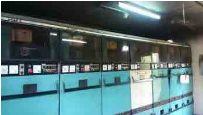
Substation (1) in Nyaung-U Town established in 1989, thus only three feeders are currently operational.
