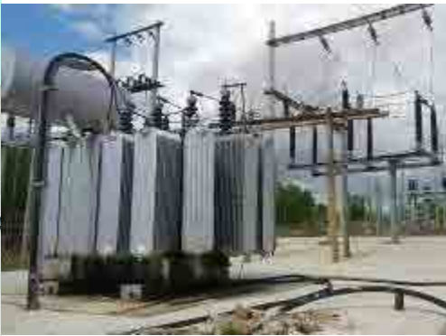
Substation in New Bagan Town
