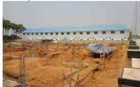
Hotel under construction in front of bus terminal. Development of bus terminal is a condition for permission for hotel construction
