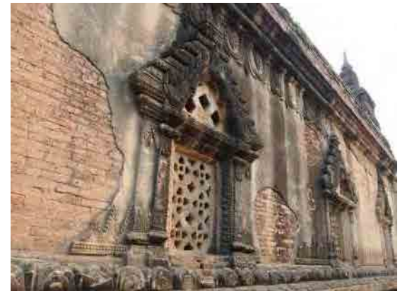
Falling of stucco on outer wall
