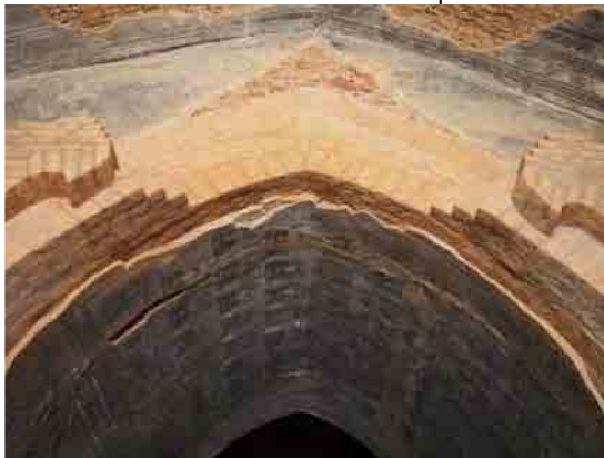
Falling of stucco on vault arch
