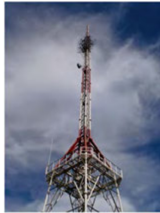
VHF Omni antenna of Nayabedda transmitting station
