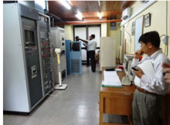
Inside of Hanthana Transmitting station of SLRC
