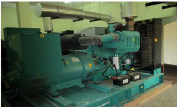
Emergency generator of Kokavil station
