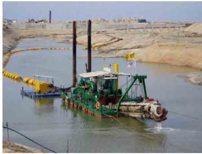
Photo 5.1 Cutter Suction Dredger
