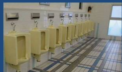
▲ Maintain clean toilet
