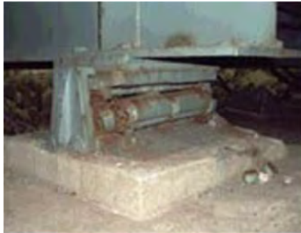
P3.7 Bearing roller dropping
