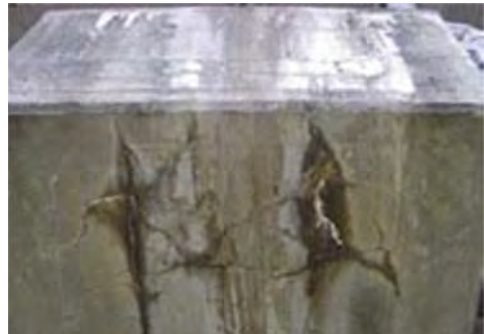
P8.10 Water from cracks and generated lime
