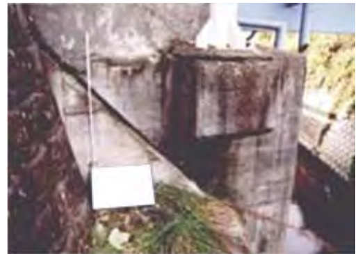
P25.4 Abutment moved
