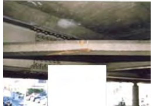
P23.8 Deformation and peeling of paint on the lower lateral bracing
