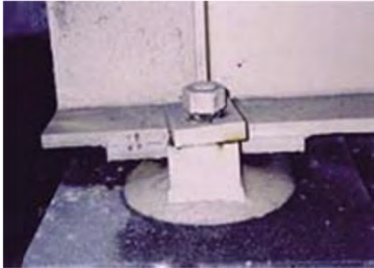
H16.7 Loosening of anchoring bolt at bearing shoe
