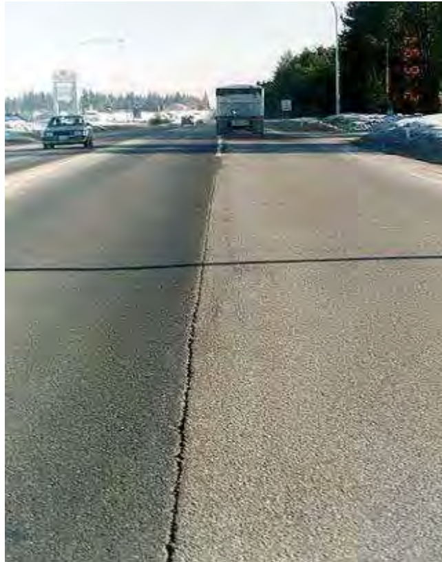
Image 5.5.11 Reflection cracks from old concrete pavement
