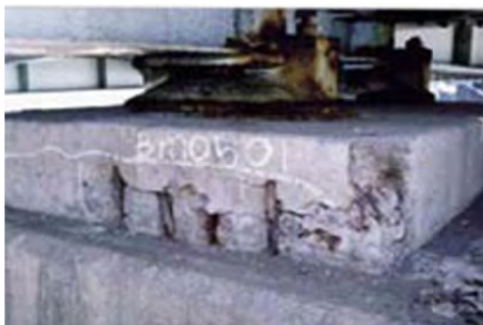
H16.11 Base concrete damage at bearing shoe
