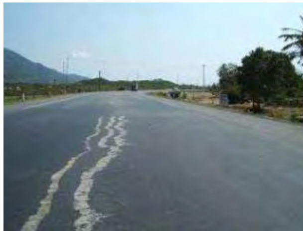
Image 5.5.1 Bleeding and fatting-up of asphalt pavement
