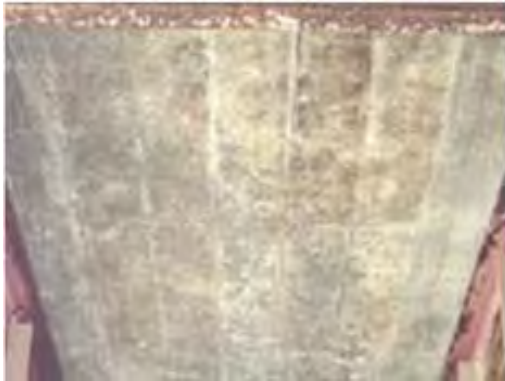
P19.1 Discolor of concrete floor
