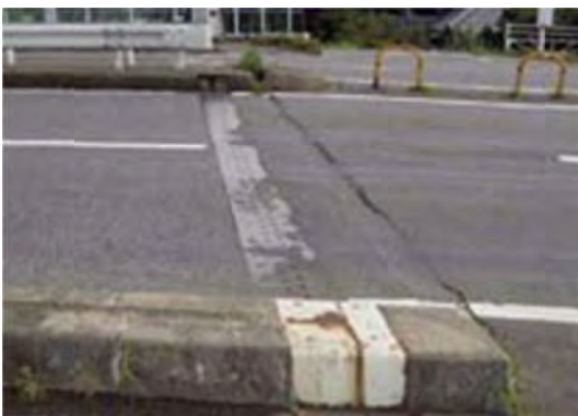
P 14.8 Damage of back up of parapet at abutment
