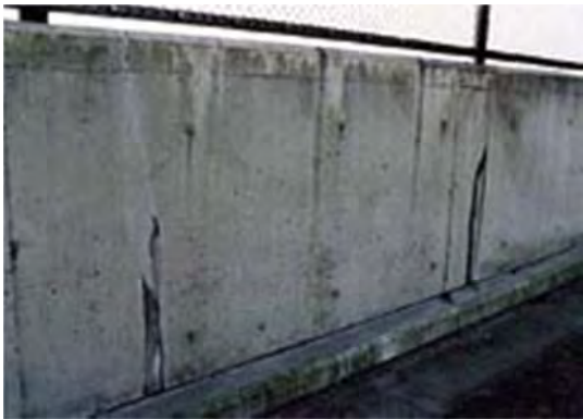
P6.3. Railing wall cracked
