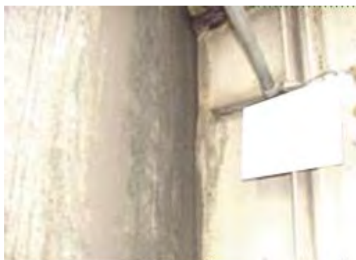
P25.6 Touching of girder and parapet
