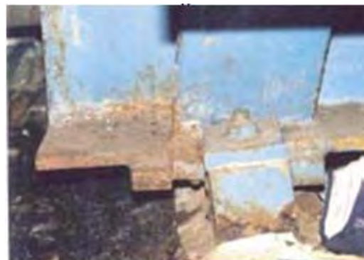
P25.9 Tilting and corrosion at bearing shoe
