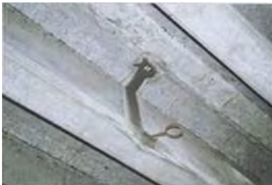
P20.10 Rapture at drain pipe
