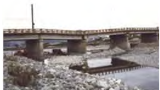
H22.2 Substructure settlement leads the extra ordinary sagging at super structure
