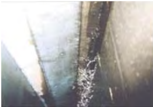
P20.1 Water leaked from expansion joint
