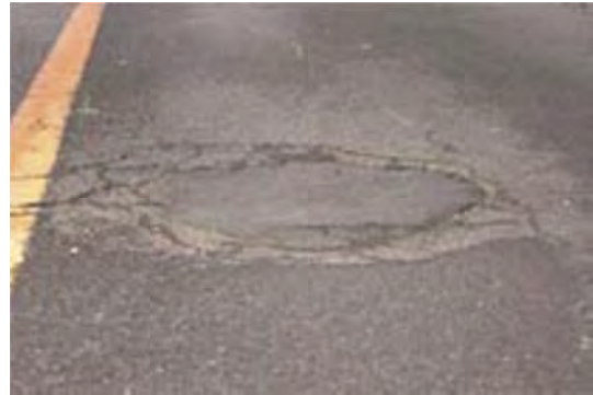
P 14.6 Cave in (Sinking) of pavement
