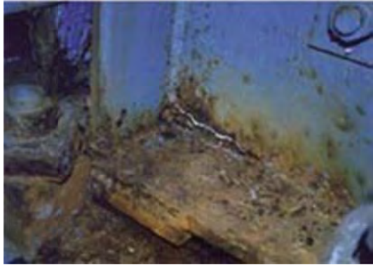
P11. Crack and corroded
