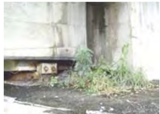
P24.4 Dumping of debris around the bearing shoe.
