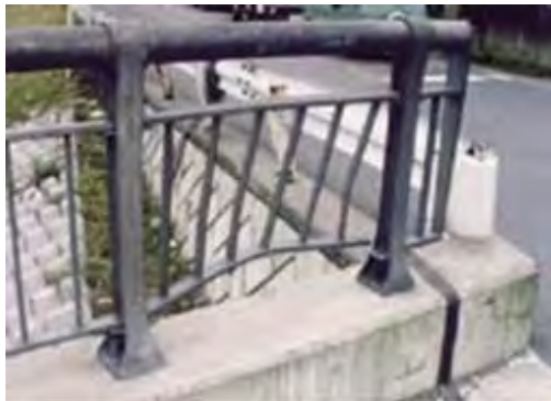
P23.9 Deformation and rapture at railing of sidewalk
