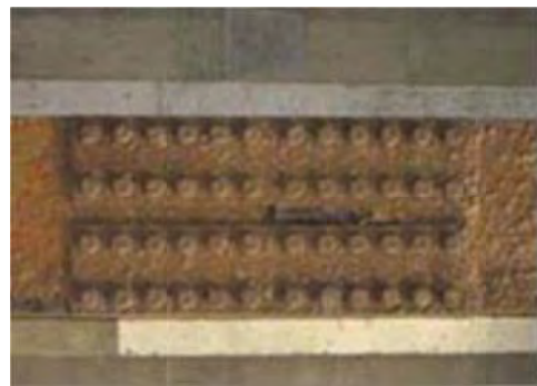
P5.6. Unstable rust on weathering steel surface
