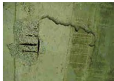
P12.10 Peeling and rebar exposure occurred at girder
