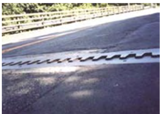
P 14.3 Extra ordinary gap at expansion joint
