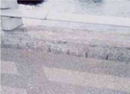
Remark: Exposure rebar but not severely corroded.
