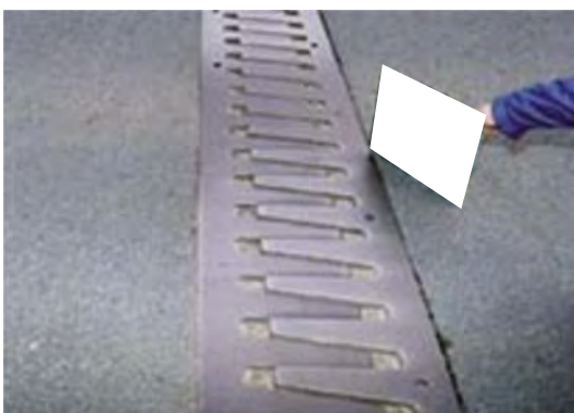
P 14.4 Extra ordinary gap at expansion joint
