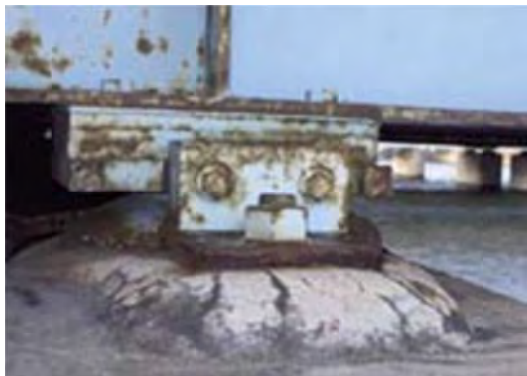
H16.9 Damage on the mortar of bearing shoe base
