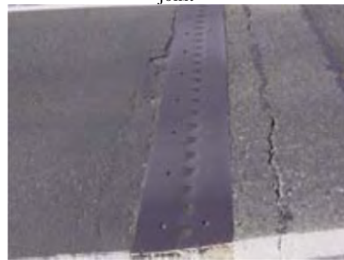
P 13.6 Cracks on pavement due to touch of expansion joint gap closure
