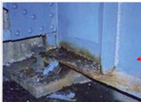
P4. Corrosion at Girder End or Bearing Shoe by water and debris
