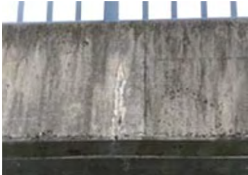
P8.1 At railing wall crack and free lime occurred between connection joint.
