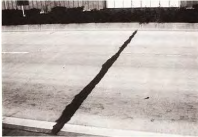
Image 5.6.6 Leaking of filler
