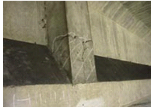
P18.8 Cracks on concrete transverse PC tendon anchoring
