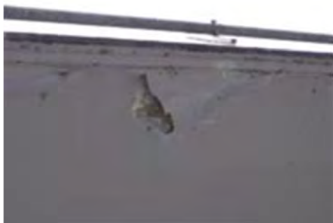
P5.11. Paint film on concrete peeled
