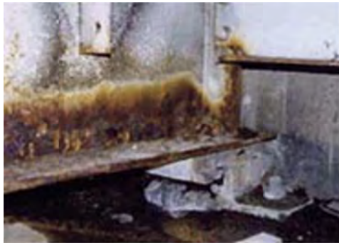
P5. Lack of Cross section
