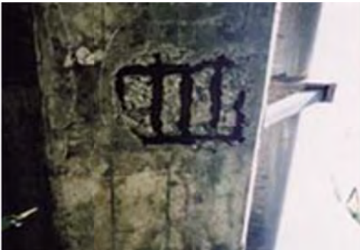
Remark: Rebar exposed and severely corroded
