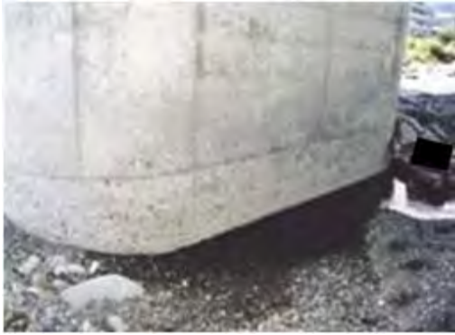
P26.1 Soil washed away at foundation
