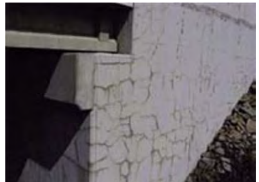
P6.6. Cracks on abutment
