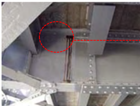
P3. Corrosion at Galvanized Steel
