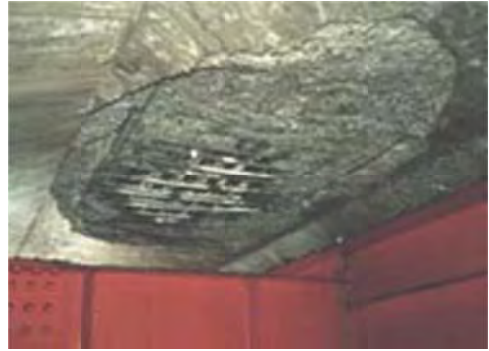
P9.2 Concrete block fall
