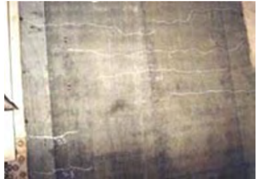
P11.2 The direction cracks at bottom of floor deck
