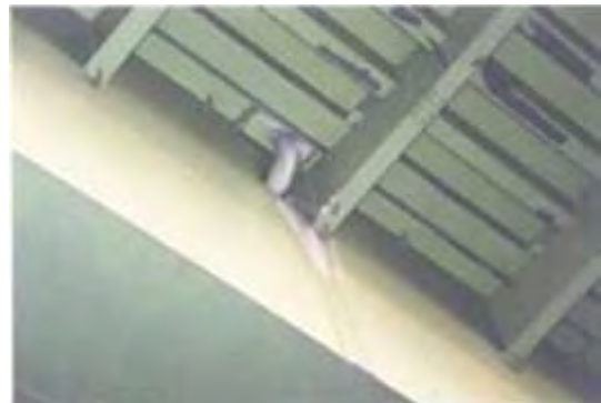
P20.2 Water leaked from drain pipe
