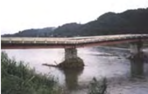
H22.1 Substructure settlement leads the extra ordinary sagging at super structure
