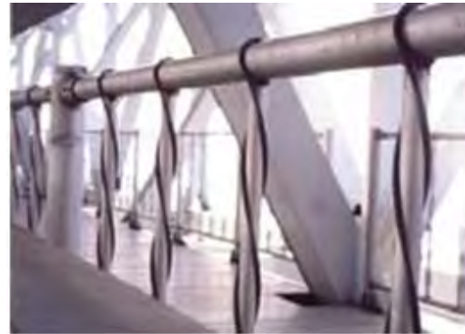
P21.4 Railing with twisted wire for vibration.
