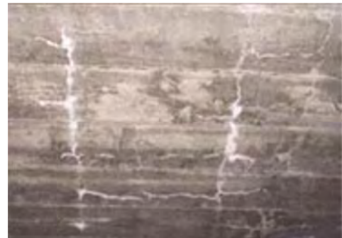
P11.10 Free lime from cracks on the bottom of floor deck
