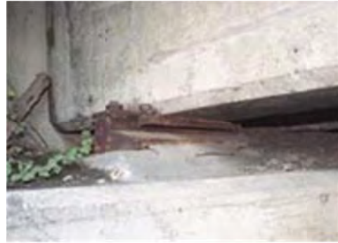
P5.8. Steel member corrosion
