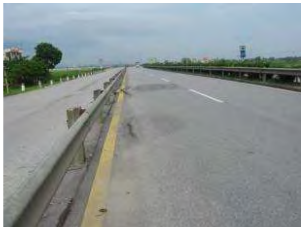
Image 5.5.17 Depression on asphalt pavement
