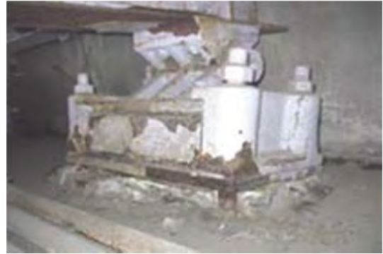
H16.2 Damaged supporting function of bearing shoe
