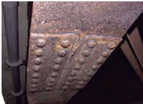
P7. Uneven corrosion and lack of cross section at weathering steel
