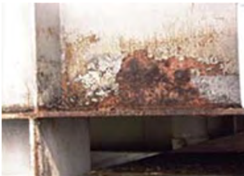
P1. Corrosion concentrated
