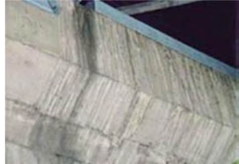
P8.8 Drained water pass through surface and generated lime
