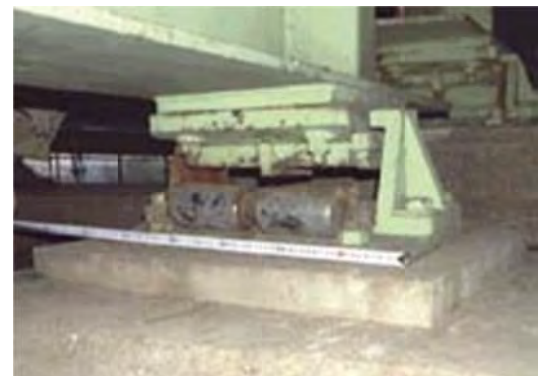
H16.6 Dropping of bearing shoe roller
