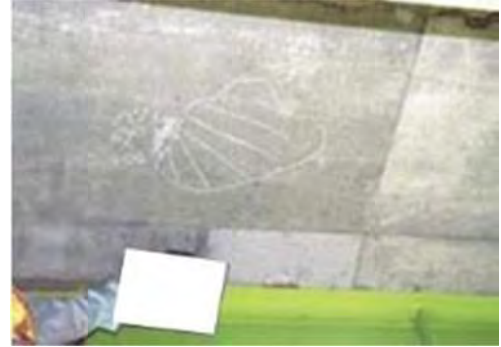
P12.2 Floating of concrete
