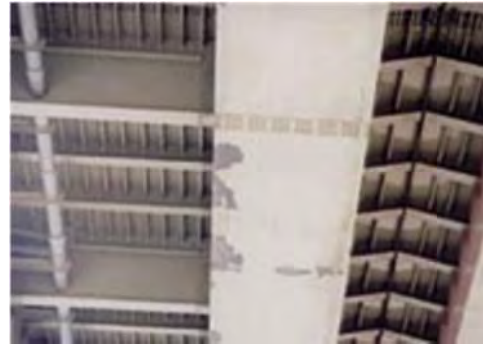
P5.2. Peeling of paint film
