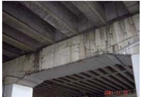
P6.4. Rigid frame pier beam cracked
