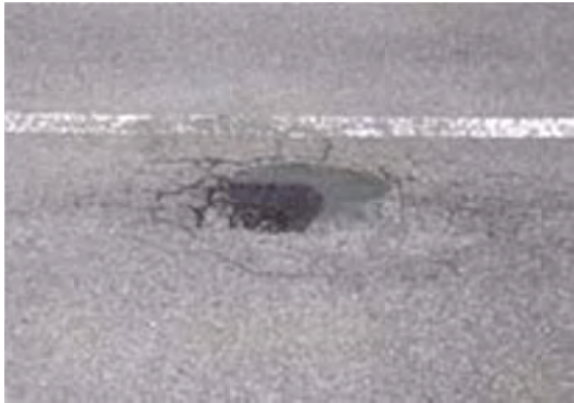
P 14.5 Pot hole on pavement
