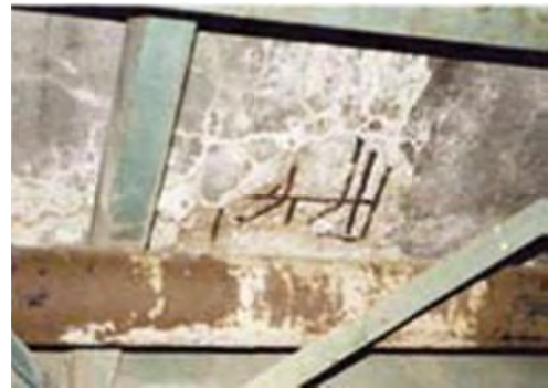
P11.8 Cracks and concrete peeling and rebar exposure on the deck bottom
