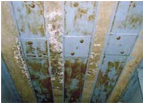
P10.5 Free lime generated at the strengthening steel plate on the bottom of floor deck
