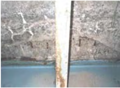
P11.7 Cracks and concrete peeling and rebar exposure on the deck bottom
