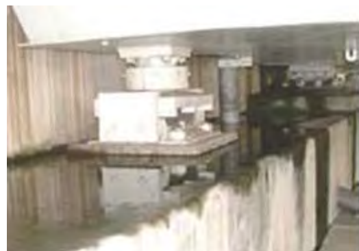
P20.5 Stagnant water at bearing shoe base
