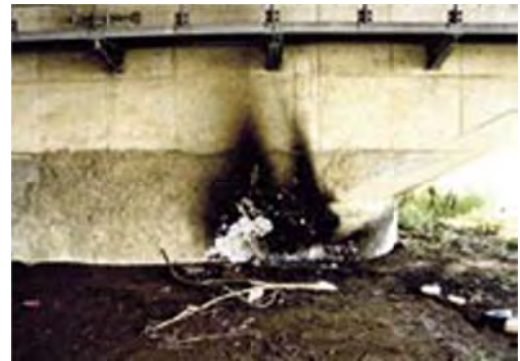
H17.4 Damage or discolor due to fire
