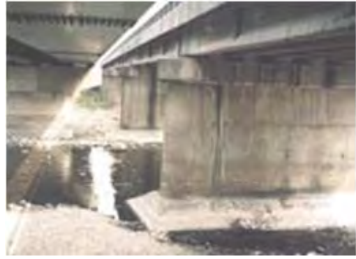
P26.2 Soil washed away at foundation
