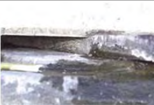
P19.3 Crack on rubber bearing shoe
