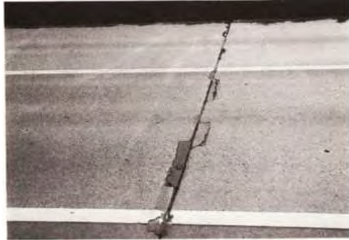
Image 5.6.7 Lost edges at the joint edge (repaired by resin mortar)
