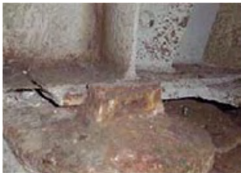
P2.8 Cross section decreased and crack occurred
