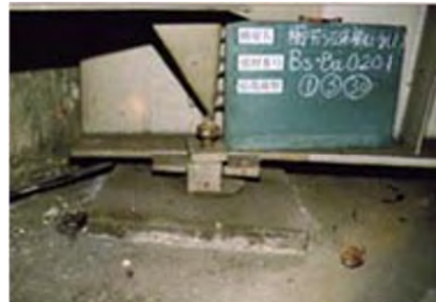
P3.8 Shoe anchoring bolt loosens
