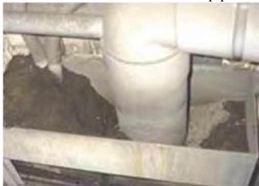
P 1: Member Catch of drain pipe
