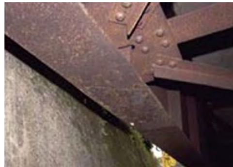
P8. Uneven corrosion but no cross section damage
