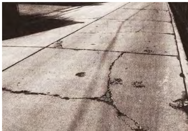
Image 5.6.11 Tortoise shell crack
