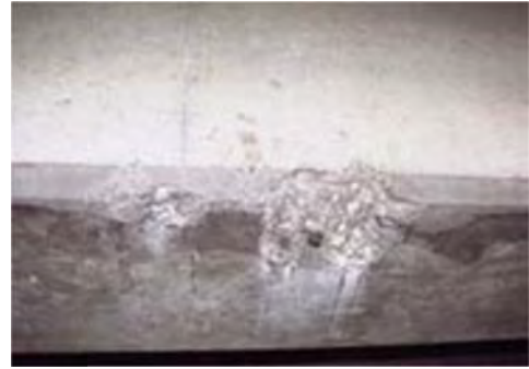
P7.8. Missing is occurred (accident occurred)
