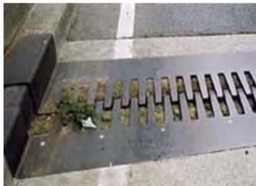
P24.5 Dumping of debris at the expansion joint
