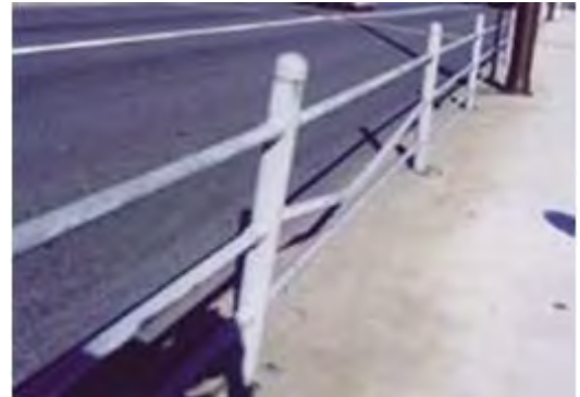
P23.4 Deformation occurred at railing
