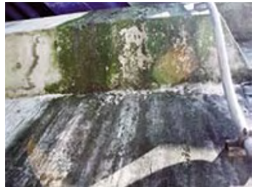
H17.6 Discolor by the flow of water on the surface
