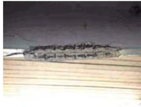
P10.8 Peelings and rebar exposure at painted girder.
