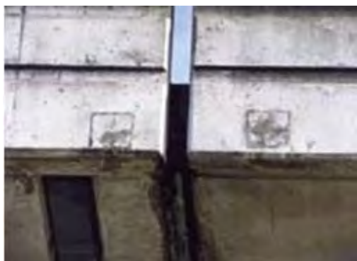
P18.1 Cracks on the anchoring concrete
