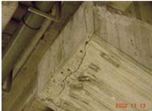
P6.7. Piling of concrete and rebar exposure and cracks
