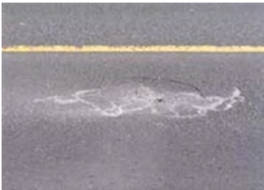
1) Damage of pavement
