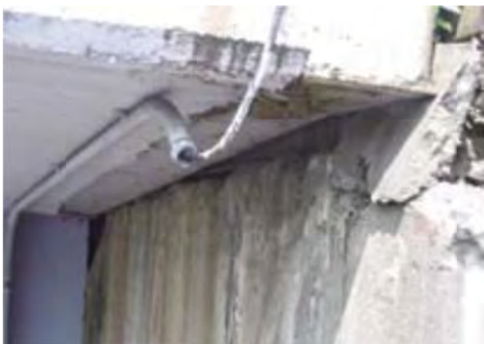
P 13.5 Parapet damaged by the floor deck and parapet touching
