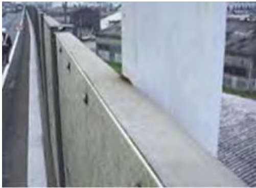
P21.1 Sound from the noise barrier and lighting pole touching
