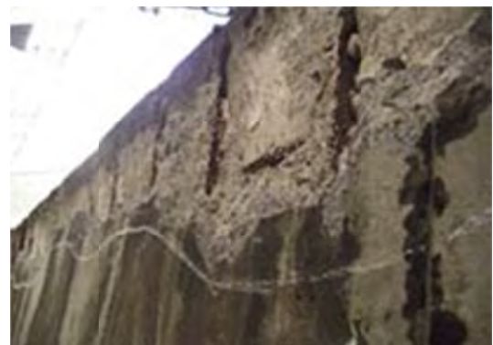
P7.6. Peeling rebar exposure
