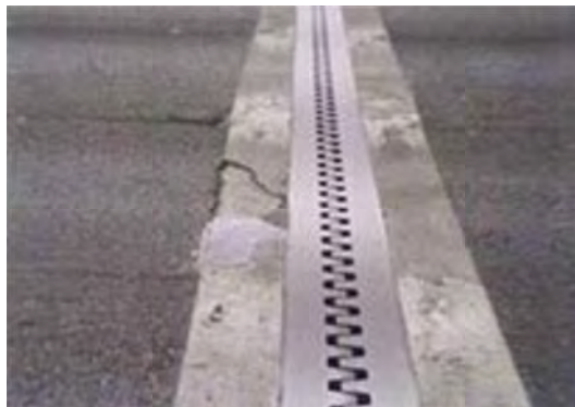
P 14.2 Gap from damage of pouring material at expansion joint
