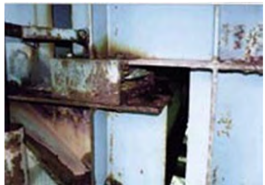
H16.4 Damage on the movement function
