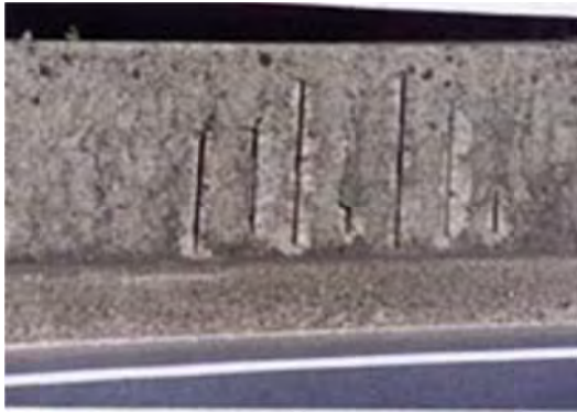
P7.1. Peeling rebar exposure
