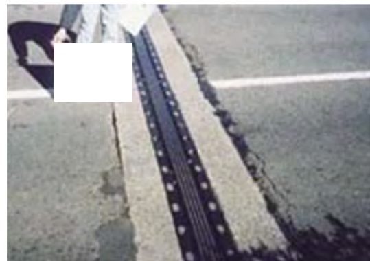
P 14.9 Gap between expansion joint and pavement
