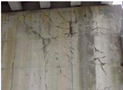
P6.5. Cracks on abutment
