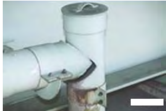
P20.9 Rapture at drain pipe
