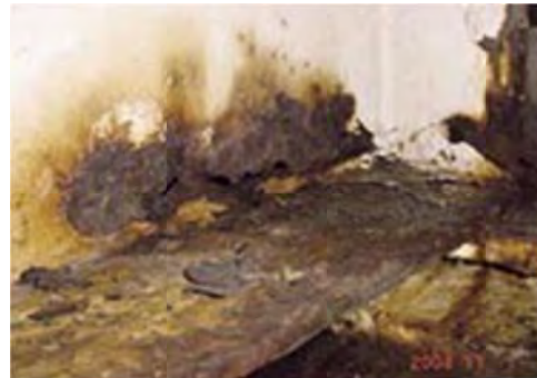
P15. Crack and lack of cross section with corrosion
