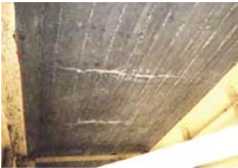
P11.9 Free lime from cracks on the bottom of floor deck
