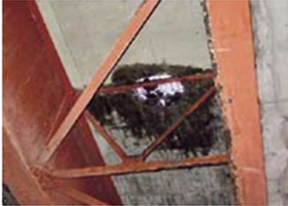
Remark: Concrete block dropping
