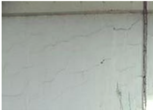
P10.7 Cracks on the painted abutment
