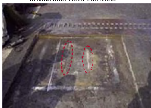
2) Steel deck cracks
