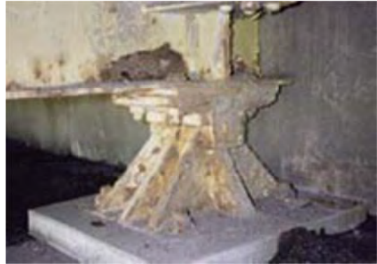
H16.8 Corrosion of anchor bolt of bearing shoe
