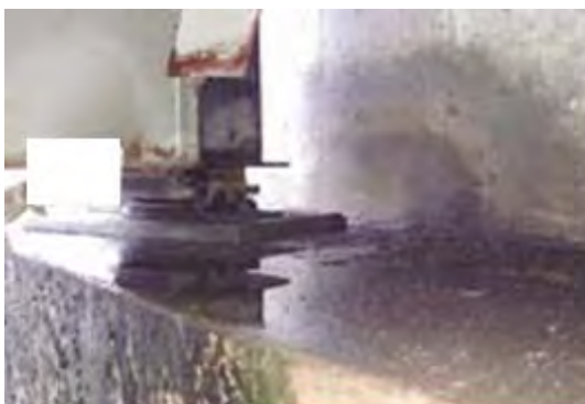
P20.4 Stagnant water at bearing shoe base
