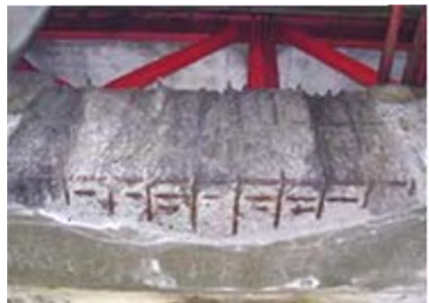
P7.10. exposed rebar is corroded and raptured
