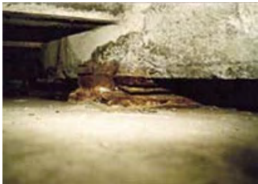
H16.3 Damaged supporting function of bearing shoe
