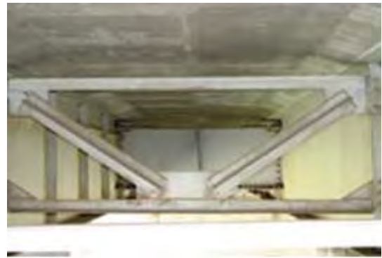
P19.6 Discolor of paint on the steel member
