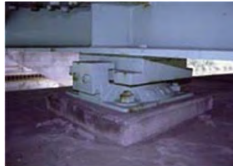
P6. Slight corrosion no cross section damage
