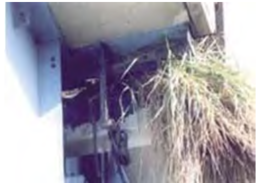
P24.6 Drain ditch is dumping of debris.
