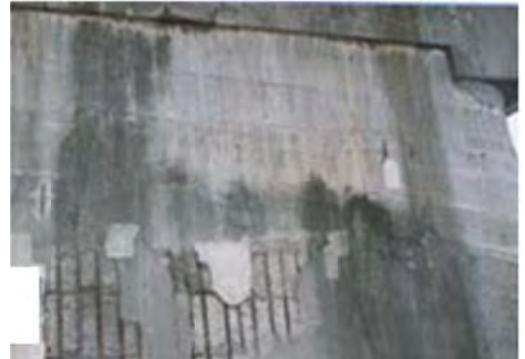
Remark: Rebar exposed and severely corroded
