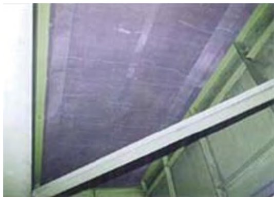
P6.9. Cracks on the floor deck
