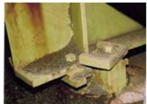
P23.6 Deformation at pinch plate of bearing shoe
