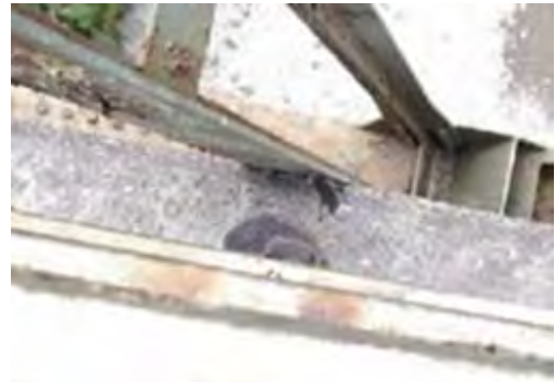
P21.2 Sound from diagonal member of truss and RC floor deck touching
