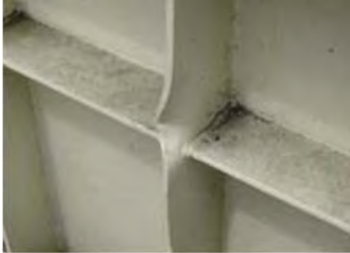
P23.1 Partial deformation at vertical stiffener
