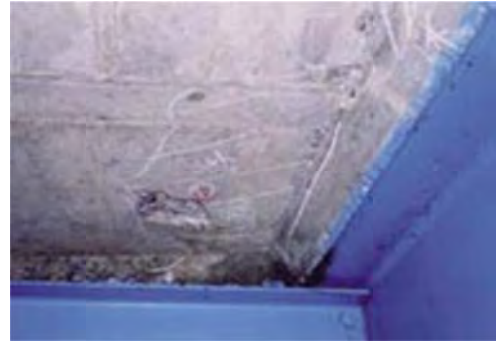
P12.8 Floating and peeling at bottom of floor deck
