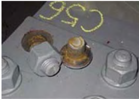
P3.3 Rapture of bolt dropping
