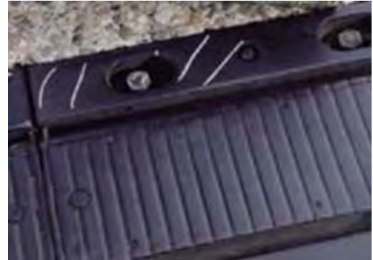
P21.6 Sound from the loosening bolt at expansion joint.
