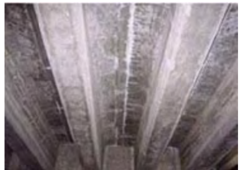
P9.5 Buffering concrete have leaking
