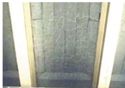
P11.6 Rectangular cracks on the bottom of floor deck
