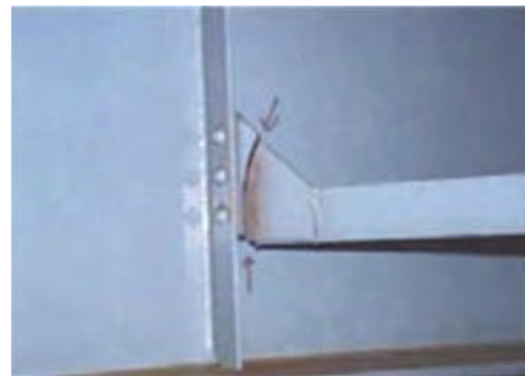
P2.9 Rapture occurred due to progress of crack
