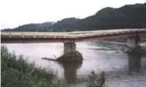
P25.3 Pier settlement
