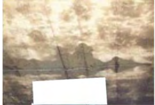
P20.7 Water leaked from crack on the floor deck
