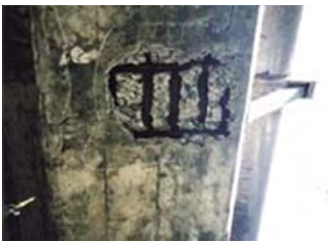
P12.9 Peeling and rebar exposure occurred at girder
