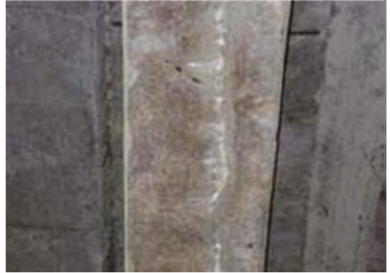
P6.2. Cracks on the girder
