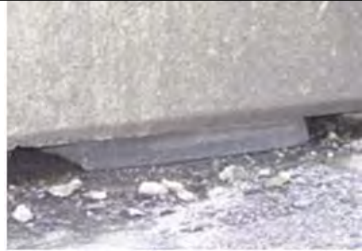
P19.4 Crack on rubber bearing shoe
