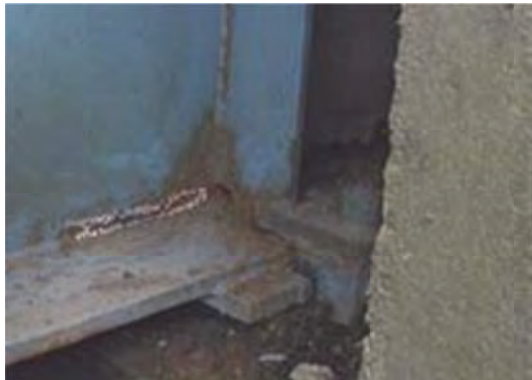
P13. Crack and corrosion
