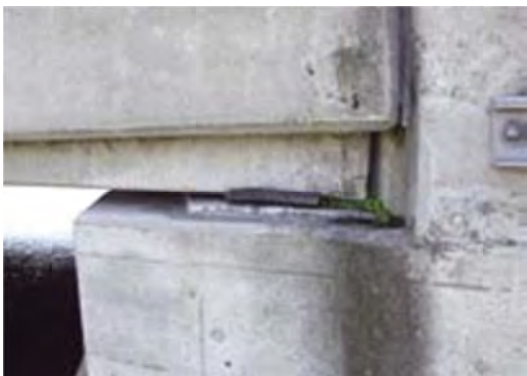
H16.5 Damages both movement and load support
