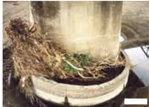
P26.4 Foundation is washed away.
