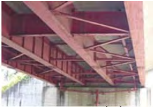
P19.5 Discolor of paint on the steel member
