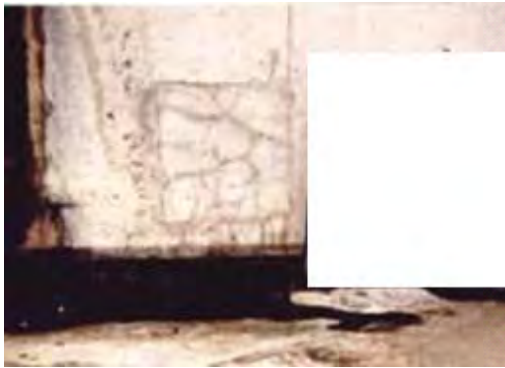
P18.7 Cracks on concrete transverse PC tendon anchoring
