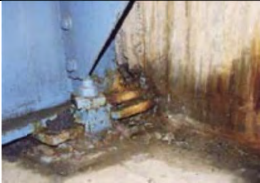
P 13.7 Bearing shoe deformation due to girder and abutment touching
