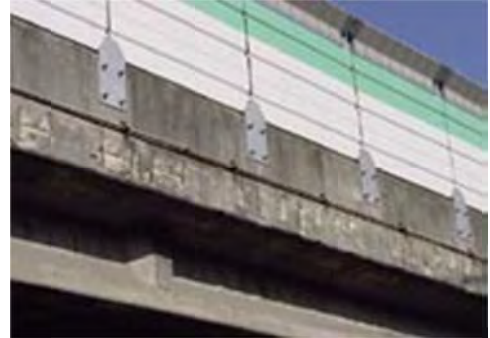
No 2: Member Backs side of curbs
