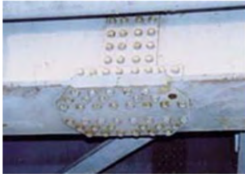
P3.1 Bolt dropping
