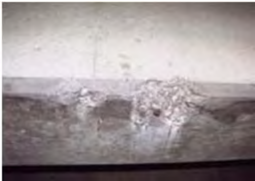
P23.3 Lack of cross section at girder
