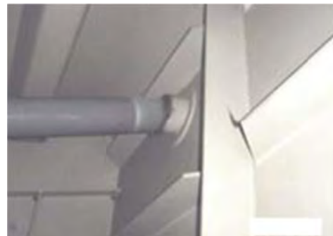
No 18: Member Girder
