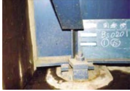
P 13.2 Touching of girder end and abutment and damage on punch plate of bearing shoe
