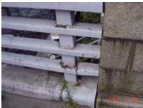
P 13.11 Railing damaged due to the gap is unusual
