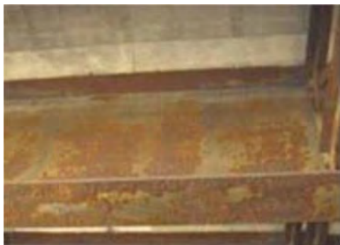
P5.5. Unstable rust on weathering steel surface
