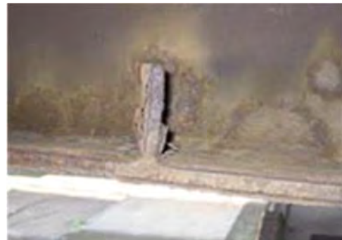
P5.10. Decrease of cross section at weathering steel
