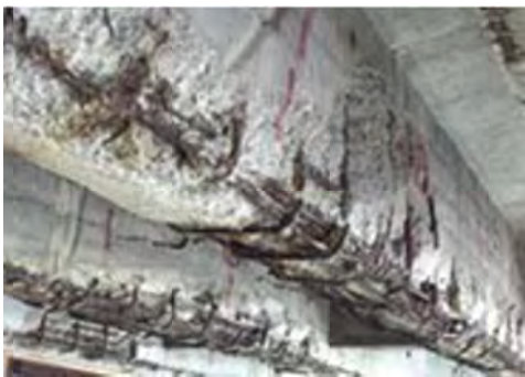
P7.9. exposed rebar is corroded and raptured
