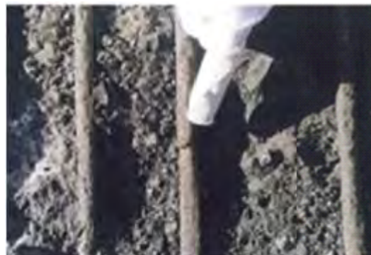
P 15.4 The upper surface of floor deck concrete changed to sand after rebar corrosion
