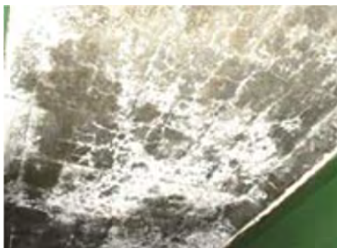
P9.4 Crocodile cracks with free lime at the reverse (bottom) side of floor deck
