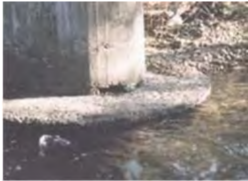
P26.3 Foundation is washed away
