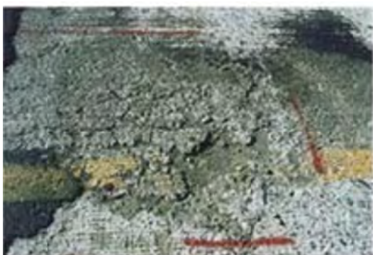
P 15.3 The upper surface of floor deck concrete changed to sand
