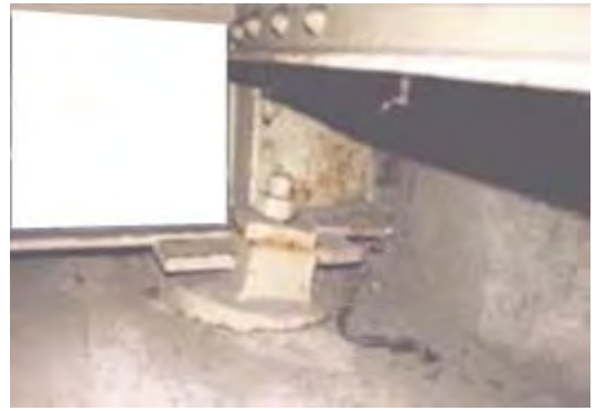
P25.2 Tilting and settlement at bearing shoe
