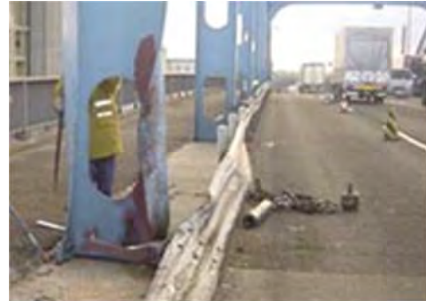
P4.6. Suspender member is ruptured as breakage and deformation.
