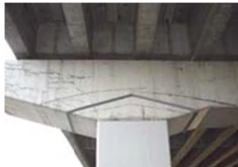
P5.12. Paint film on concrete deteriorated
