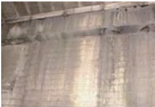
P19.7 7 Discolor of concrete surface by flow of water
