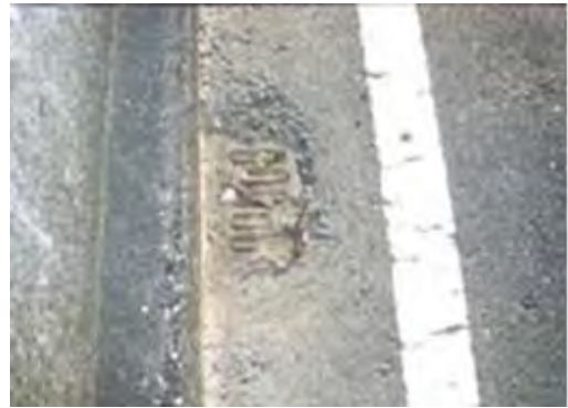
P24.2 Catch basin has dumping of debris.
