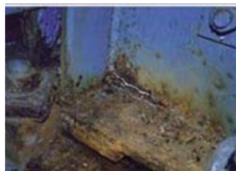
P2.5 Crack with rust
