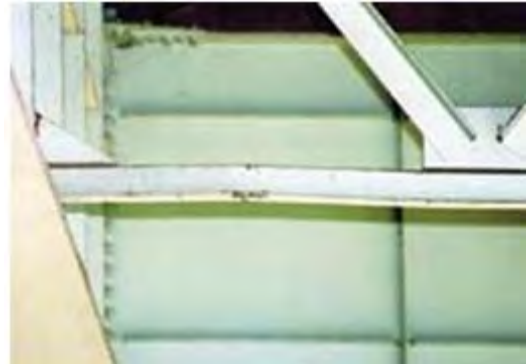
P23.2 Lateral bracing have partial deformation
