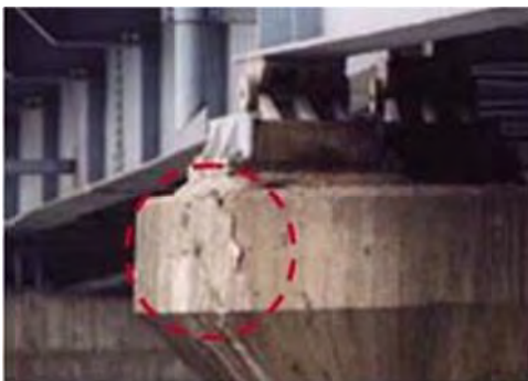
P12.5 Floating of concrete
