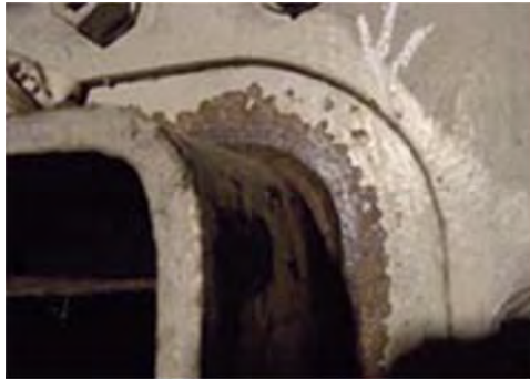
P2.1 Crack on R shape area at girder end
