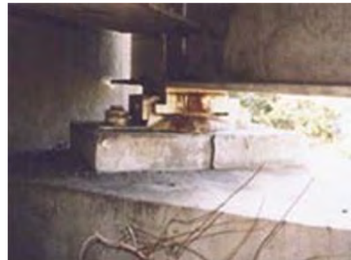
H16.12 Base concrete damage at bearing shoe
