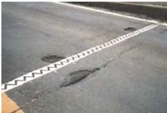
P 14.1 Gap due to pavement failure
