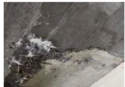
P9.9 Free lime and crack with leaking at the floor deck
