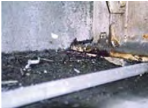
P24.3 Dumping of debris around the bearing shoe.
