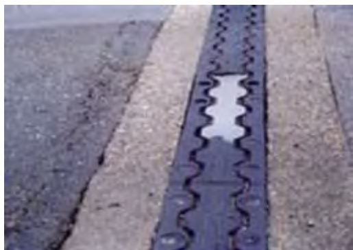
P23.5 Missing of rubber top at expansion joint
