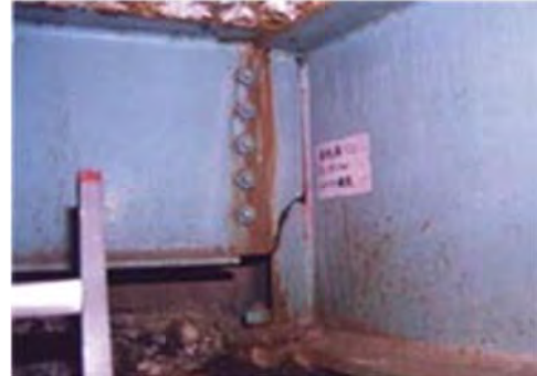
P4.2. End bracing (cross beam) has ruptured
