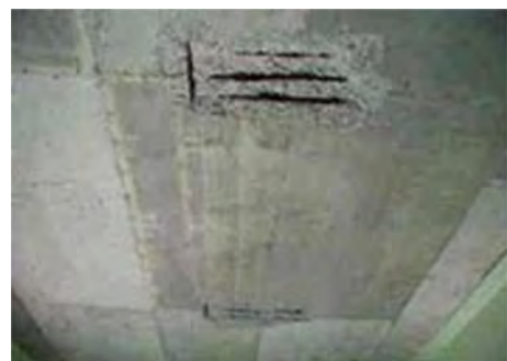
P7.12. Peeling and rebar exposure at deck floor
