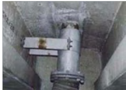
P5.4. Rust on galvanized surface
