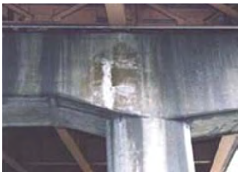
P8.5 Free lime at rigid frame pier from crack
