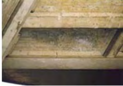
P19.2 Discolor of concrete floor
