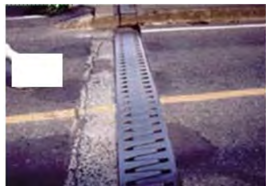
P25.7 Cracks on the back up of expansion joint
