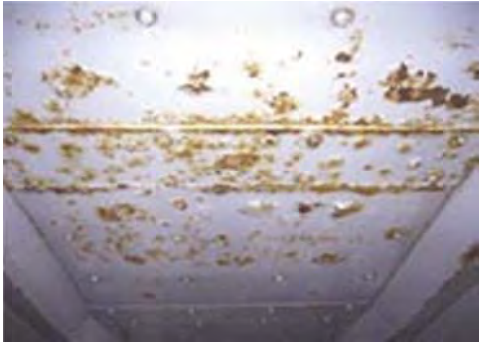
P10.1 Corrosion on the strengthening steel plate at the floor deck bottom
