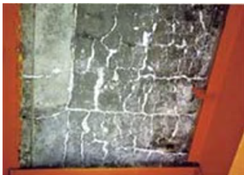
P11.11 Water leaking and free lime from cracks on the bottom of floor deck
