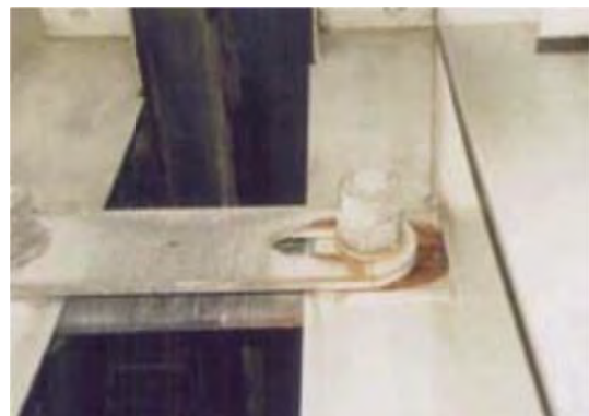
P 13.10 Movement of connection plate has deviation
