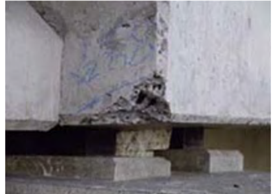
Remark: Exposure rebar but not severely corroded.
