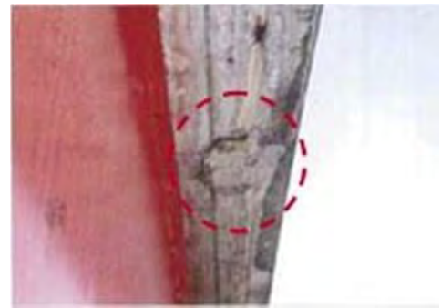
P12.4 Floating of concrete
