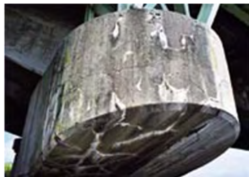
P8.6 Free lime come from crack at T shaped pier
