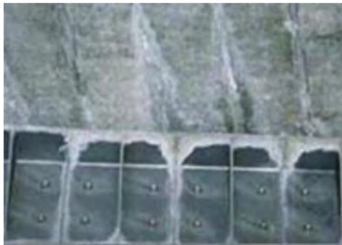
P5.3. Discolor on galvanized surface
