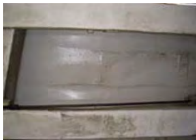
P9.8 Damage on the floor deck with strengthening
