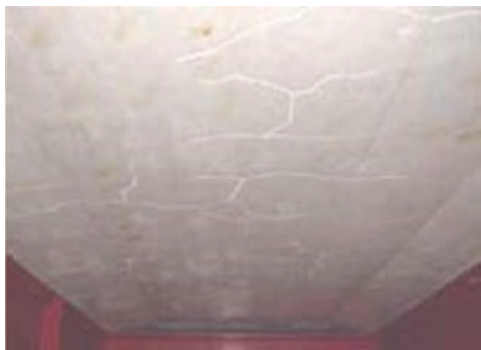
P11.3 Direction cracks at the bottom of floor deck
