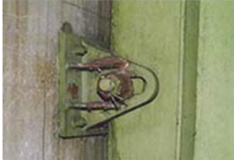
No 13: Member Bridge corruption
