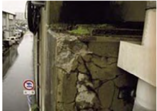
P6.8. Peeling of concrete and cracks
