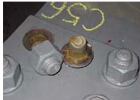
P4.8. Bolt rupture
