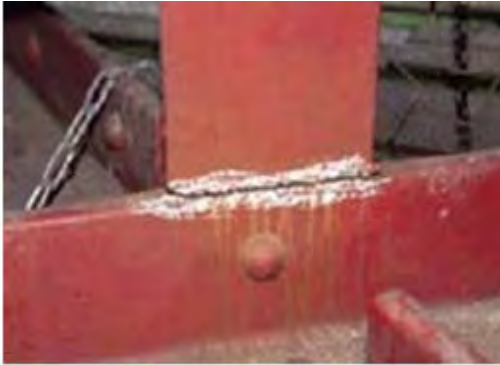
P21.5 Sound from the rupture portion between bracing and suspender connecting weld
