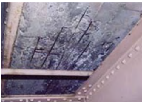
P7.11. Peeling and rebar exposure at deck floor
