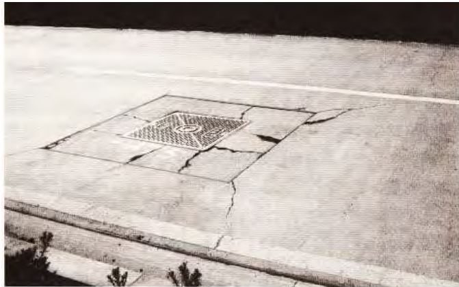
Image 5.6.1 Cracks near manhole
