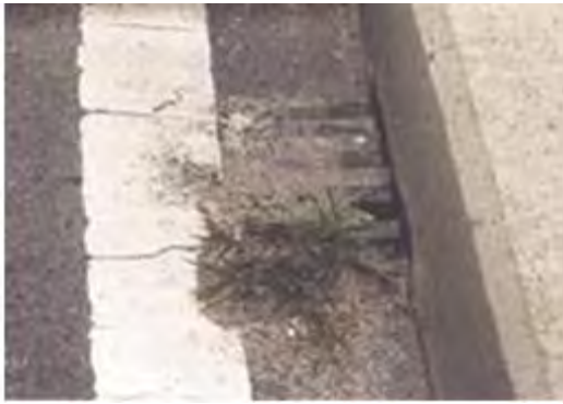
P24.1 Catch basin has dumping of debris.
