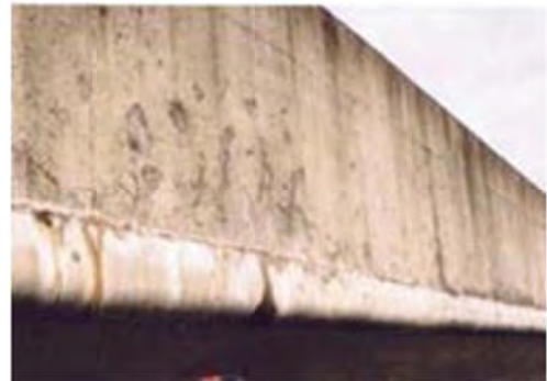
P8.2 Cantilever floor deck and curb free lime generated.
