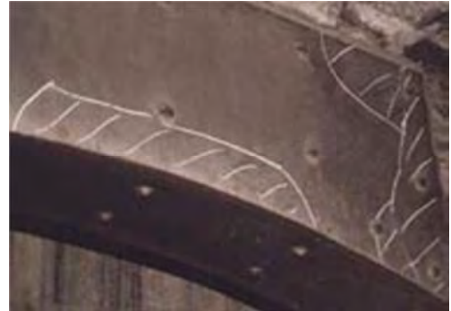
P10.2 Floating of strengthening steel plate at the girder
