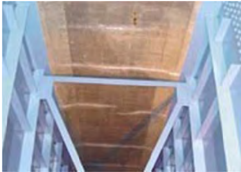
P11.1 The direction cracks at bottom of floor deck
