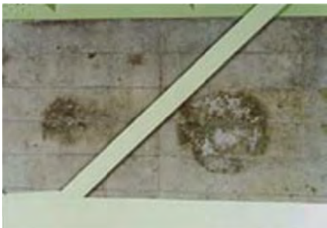
P8.11 Leakage at floor deck
