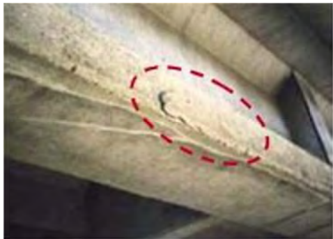
P12.3 Floating of concrete
