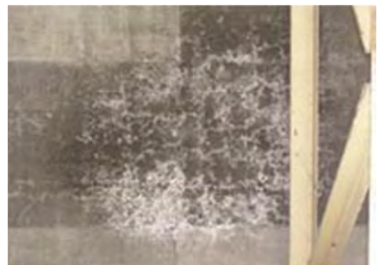
3) Cracks and free lime at bottom of floor
