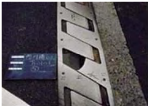
P4.3. Expansion joint finger ruptured
