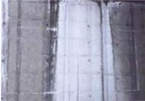
P8.7 Drained water pass through surface and generated lime
