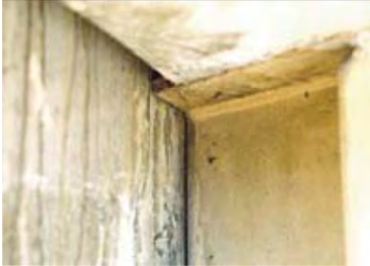
P 13.1 Touching of girder end and abutment
