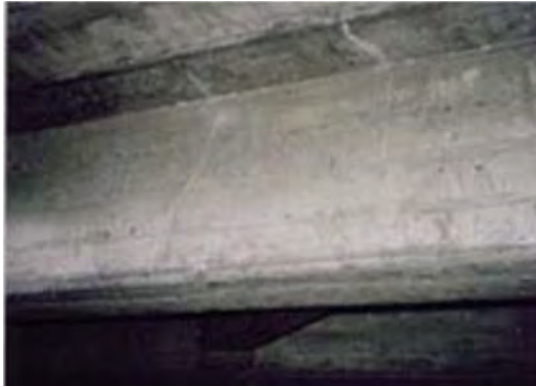
P6.1. Cracks on the girder
