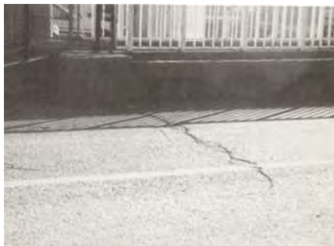
Image 5.5.13 Grade Depression at Structures
