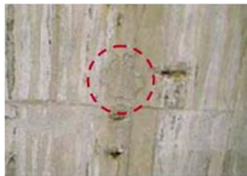
P12.6 Floating of concrete
