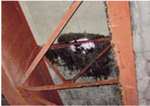
P9.1 Concrete block fall
