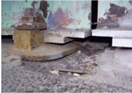
H16.1 Damaged supporting function of bearing shoe
