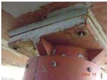
Raptured at set bolt P3.9 After earthquake
