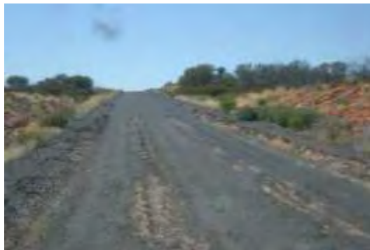
Image 5.5.3 Raveling of asphalt pavement
