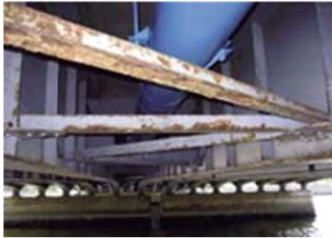
P5.7. Steel member corrosion
