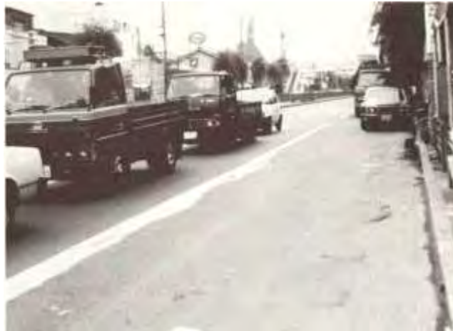
Image 5.5.16 Shoving of asphalt pavement
