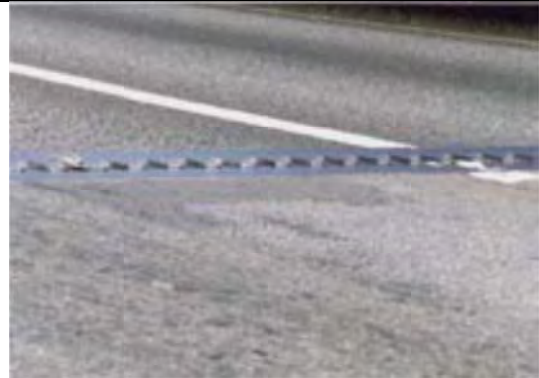
P 13.8 Gap of surface at expansion joint
