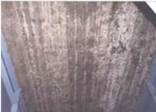
No 5: Member Floor deck
