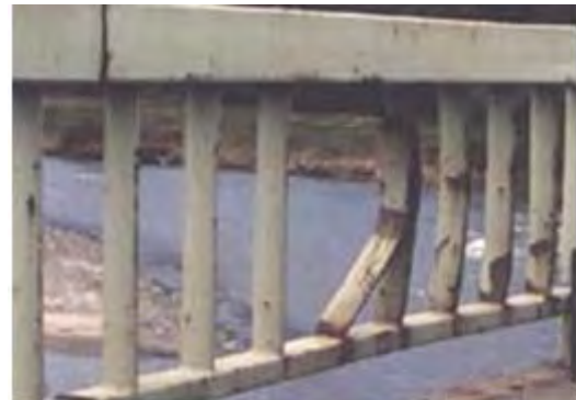
P23.10 Deformation and rapture at railing
