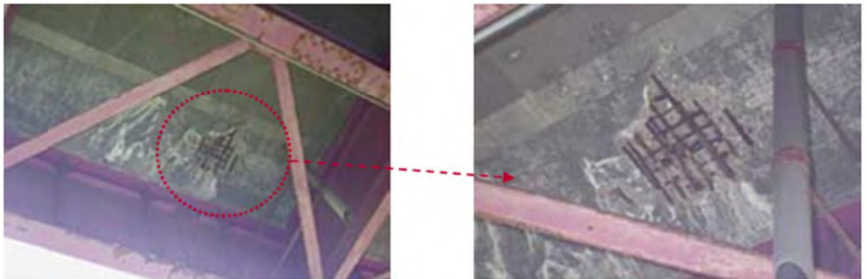
P9.7 Concrete peelings at floor deck bottom
