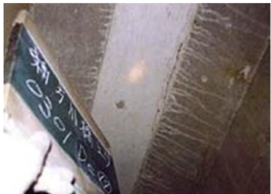
P6.10. Cracks on the floor deck between girders
