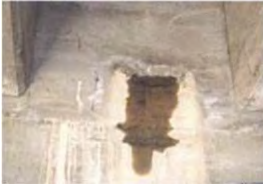
P20.6 Water leaked from abutment concrete break
