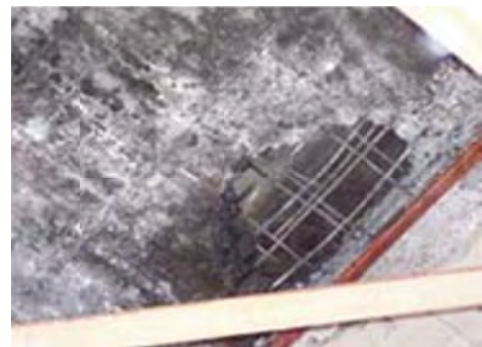
P11.12 Dropping of concrete block at the bottom of floor deck
