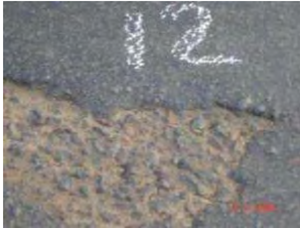
Image 5.5.2 Fretting and stripping of asphalt pavement
