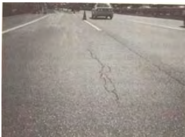
Image 5.5.8 Longitudinal single crack
