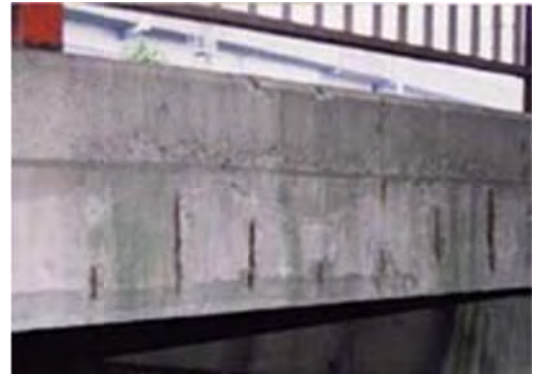
P7.2. Peeling rebar exposure
