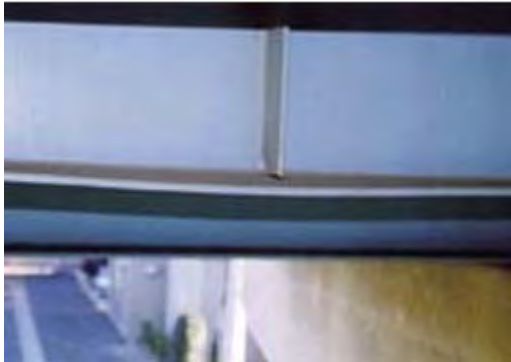
P23.7 Deformation and crack on the lower flange of stringer
