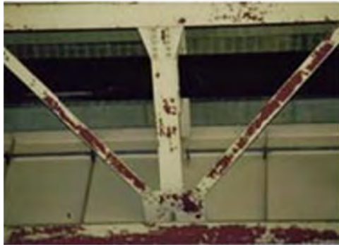
P5.1. Paint film deterioration with corrosion
