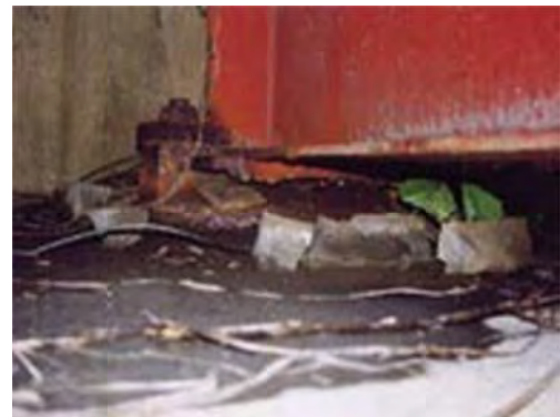
H16.10 Damage on the mortar of bearing shoe base
