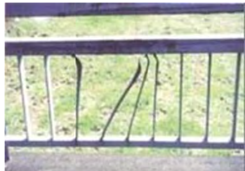
P4.4. Railing has ruptured
