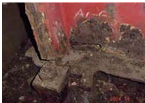
P14. Crack and lack of cross section with corrosion
