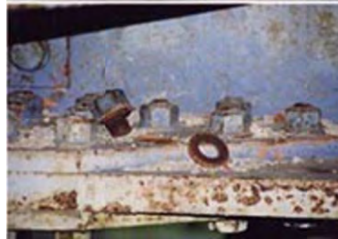
P3.4 Bolt dropping
