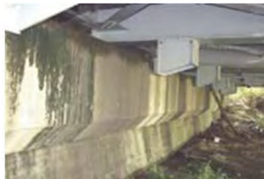
P19.8 Discolor of concrete surface by flow of water
