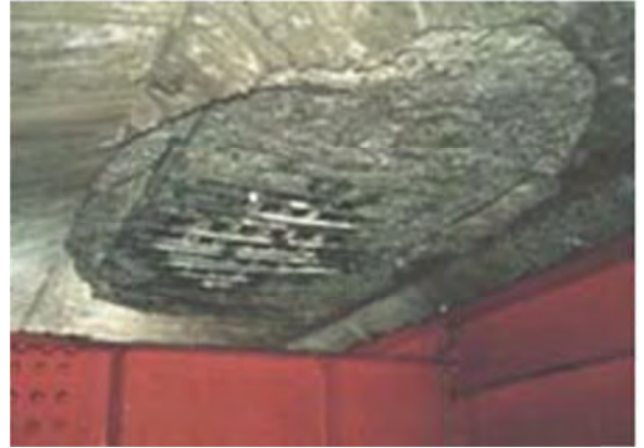
Remark: Concrete block dropping
