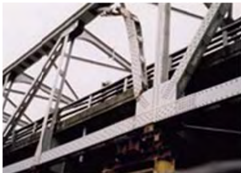
P4.7. Diagonal rupture and deformation
