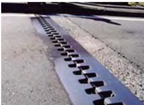
P25.8 Vertical gap and wide gap at the expansion joint
