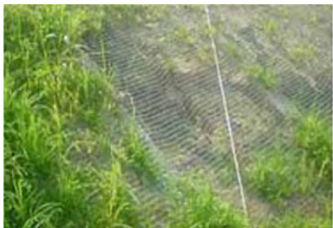
Photo 2.3 Embankment material is washed away due to weakened slope end and spring water.
