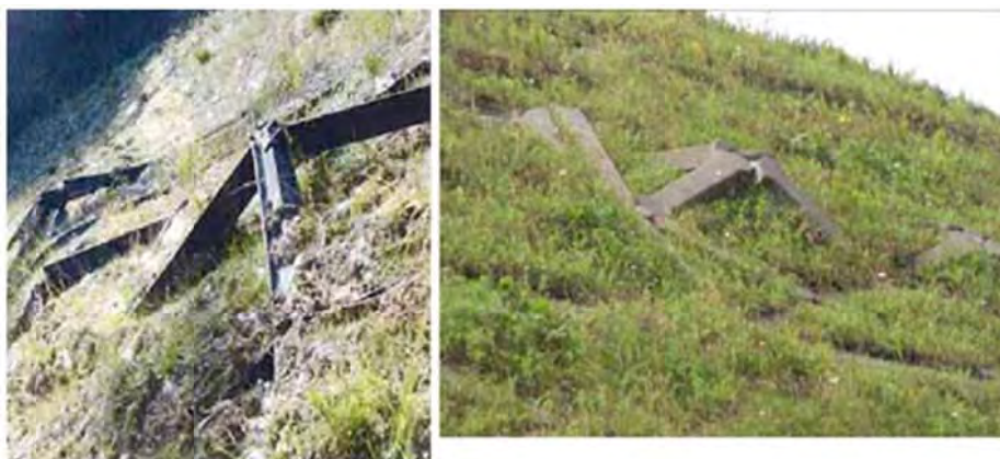
Photo 6.7 Example of deformation of frame (Rank E)
