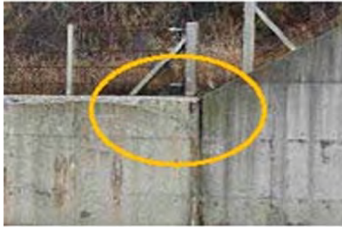
Photo 5.5 Peeling, crack on concrete (retaining wall)
