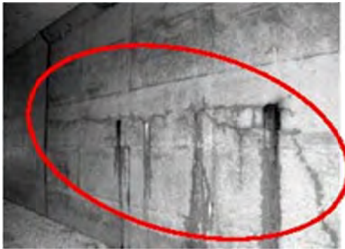
Photo 6.1 : Crack from freezing
