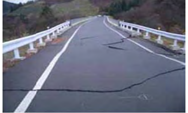
Photo 7.9 Road surface settlement
