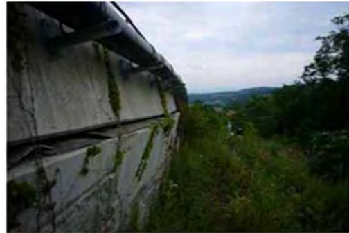
Photo 4.2 Tilting of retaining foundation
