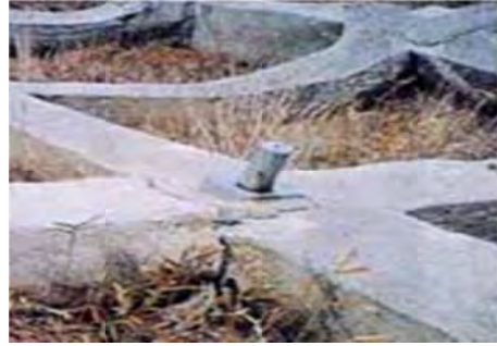
Photo 3.2 Failure of passive earth pressure structure
