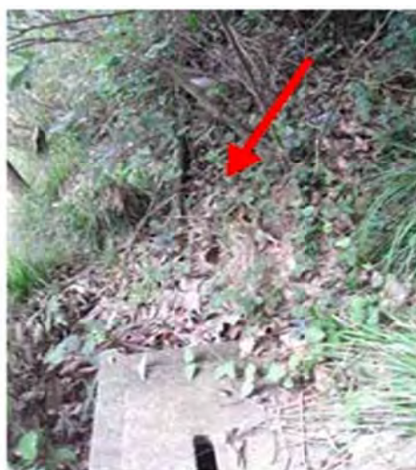
Photo 6.9 Drain ditch malfunctioning Rank D. Should be cleaned.
