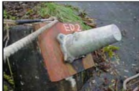
Photo 7.5 Anti-rust oil leaking
