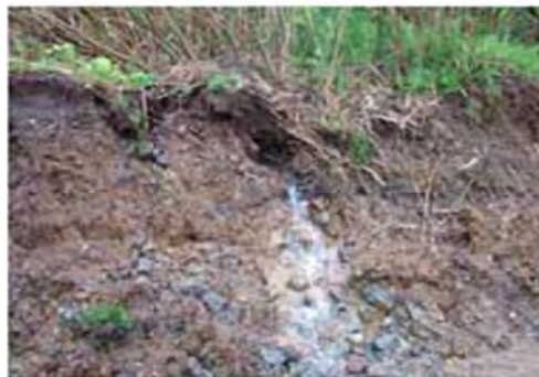
Photo 2.4 Slope and failure and spring water
