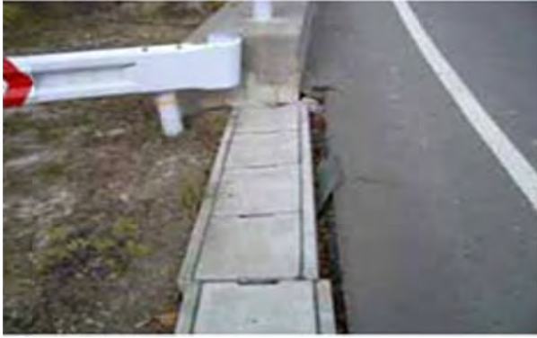
Photo 7.8 Drain system malfunction
