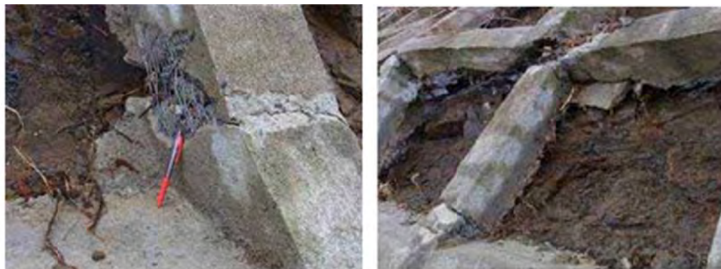
Photo 6.5 Slope protection frame breakage
