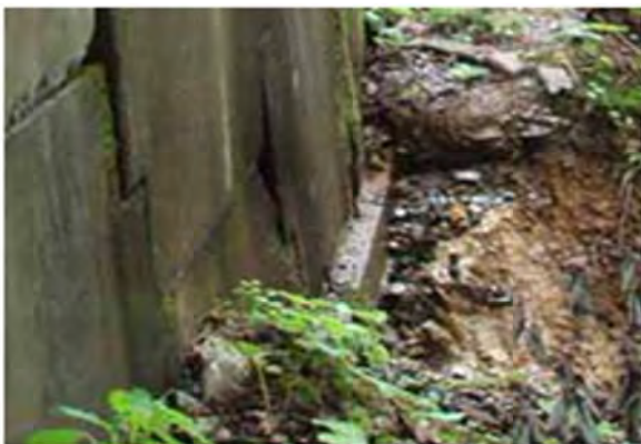
Photo 7.6 : Scouring of base foundation
