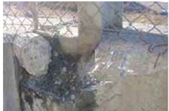
Photo 5.4: Concrete peeling, cracks (retailing wall)
