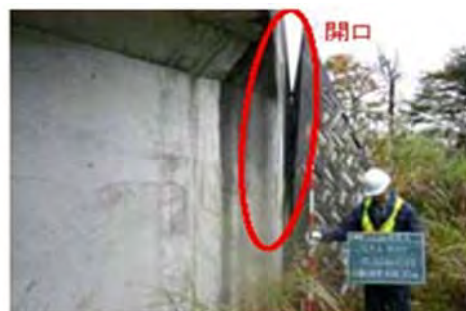
Photo 7.13 : Example of peeling, floating, cracks at the wing section
