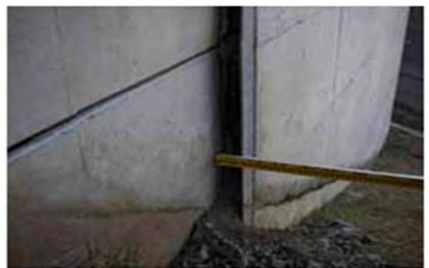
Photo 7.7 : Joint opening and sediment flow
