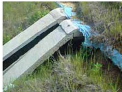
Photo 2.2 Drain system failure due to slope settlement
