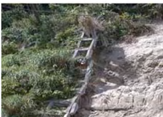
Photo 6.6 Example of crack on the slope protection frame
