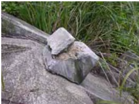
Photo 3.3 Failure of concrete head
