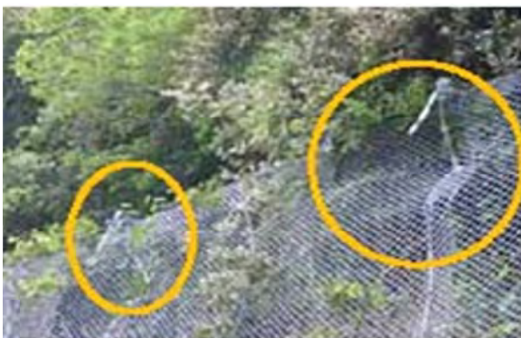
Photo 5.3 Rock fall prevention net, (pylon tilting net rapture wire rope breakage)
