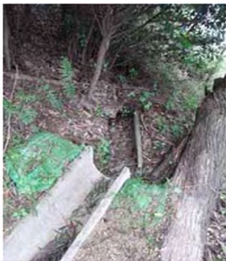
Photo 6.8 Drain ditch gap Rank E and it should be repaired.
