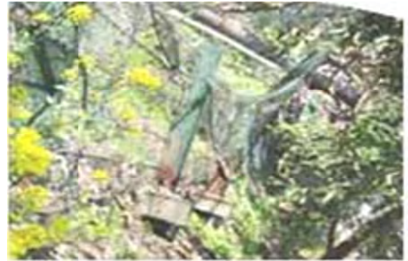
Photo 5.2: Member deformation and tilting (Rock fall prevention)
