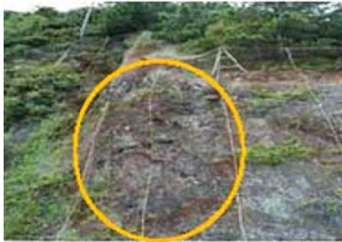
Photo 5.7 Corrosion and rapture of steel member (rock fall prevention net)
