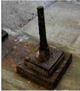
Photo 7.2 Corrosion of bearing plate
