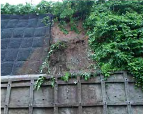
Photo 6.3 Upper slope failure
