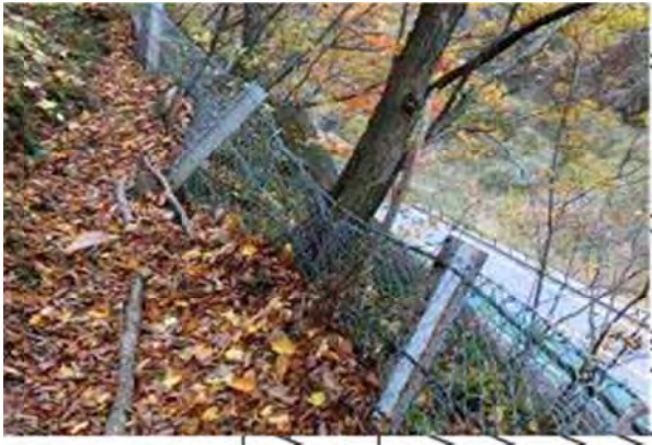
Photo 5.1 Member deformation and tilting (Rock fall prevention)
