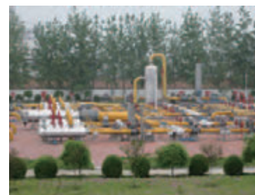
Gate stations receiving supplies of natural gas from the main pipeline (Zhumadian)
