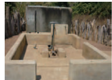
Foot-pumped deep wells with iron remover
