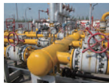
Pipeline, meters, and gauges used to make adjustments to gas pressure (Jiaozuo)
