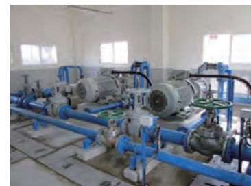
Adasiya pumping station
