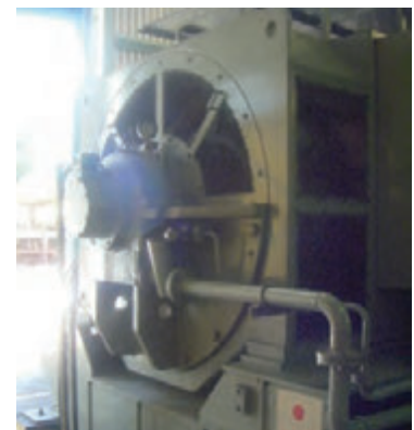
Installed Diesel Engine Generator (Lungga Power Station)
