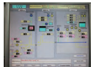
Monitor of the SCADA System
