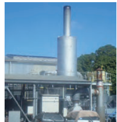
Exhaust Tower (Lungga Power Station)
