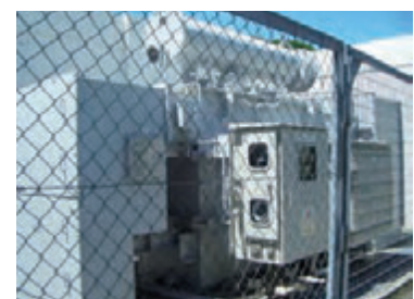
Transformer in Ranadi S/S (Ranadi Substation)
