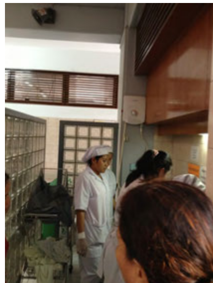
Electric water heater at the hot-water supply point
