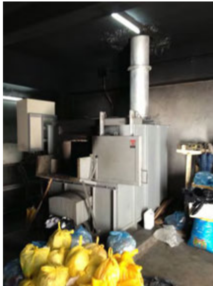
Overall view of incinerator
