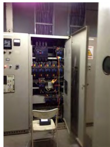
Low tension feeder board (electricity measurement underway)
