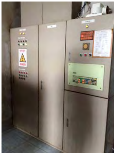
MDF and alarm board in the Security Room
