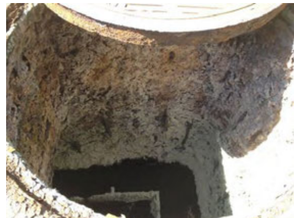
Corroded sedimentation tank
