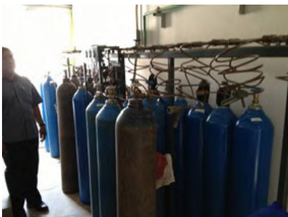
Existing oxygen gas manifold
