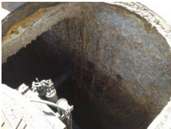
Corroded effluent pump tank
