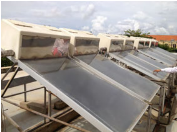
Installed solar water heaters
