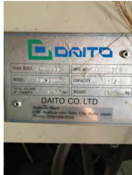
Nameplate on the incinerator
