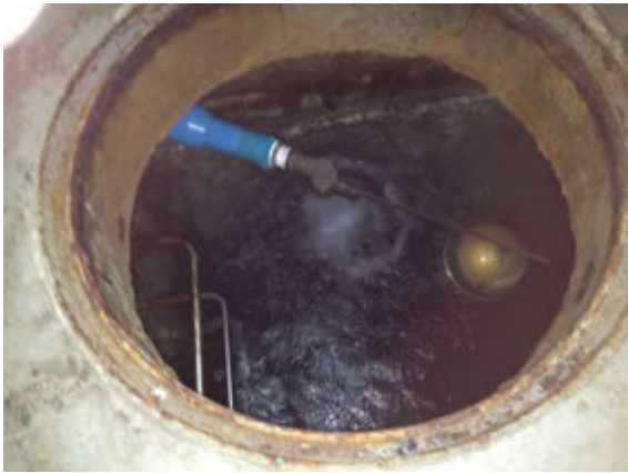
City water reception tank
