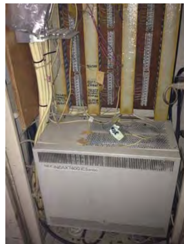
Existing private branch exchanger
